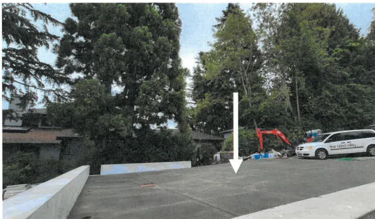
3645 Evergreen Point Rd. – One 24" Deodar cedar removed without prior consent. New driveway in location of tree (arrow). No tree protection around preserved trees as recommended by project arborist and shown in application. Revision of Administrative Tree Activity Permit application requested prior to approval.
