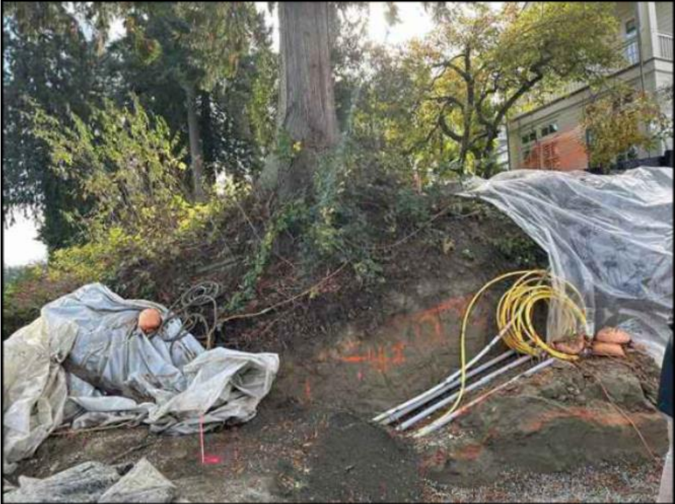
Picture 4. 3444 EVERGREEN POINT RD – High-risk western redcedar due to conditions of slope.
