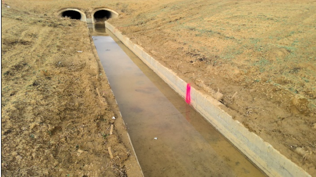
13- Crack needs replaced on trickle channel- roughly 40' south of harvest moon
