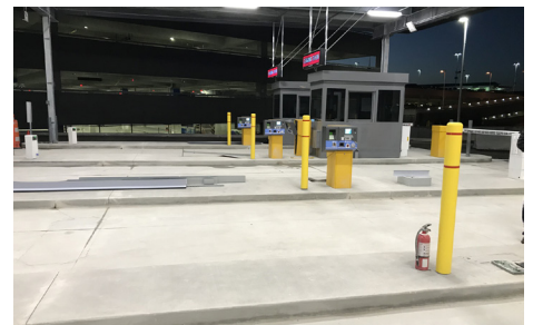
Nashville International Airport PARCS Replacement I Nashville, TN
