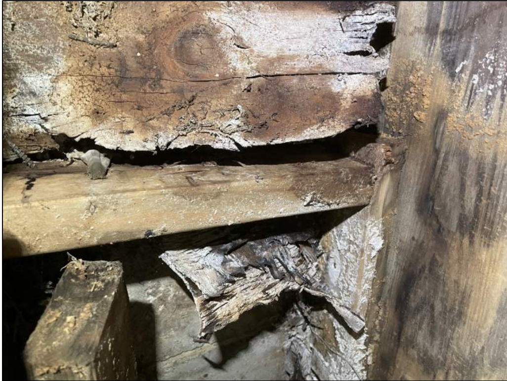
Photo 1 – Damaged or Failed Subfloor
