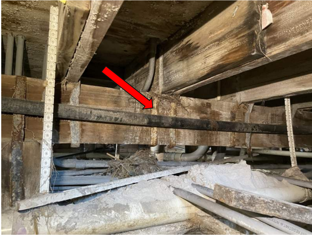
Photo 5 – Floor Joist Strap Corrosion
