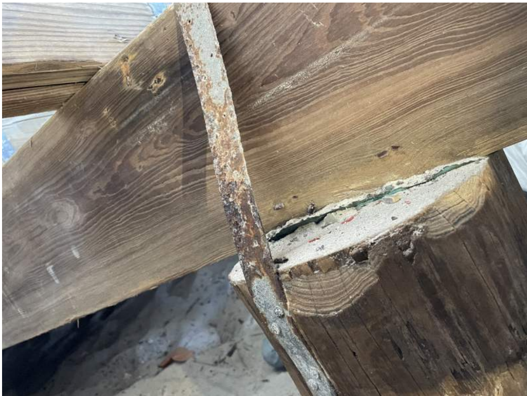
Photo 6 – Beam Strap Corrosion
