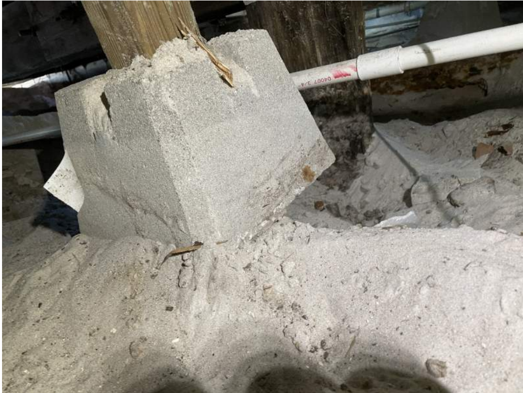
Photo 11 – Previous Retrofit Pier with Minimal Bearing on Grade
