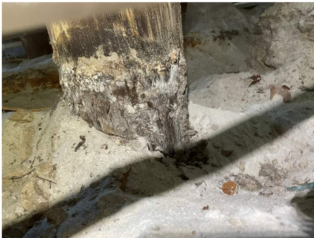
Photo 9 – Timber Pile Cross Section Loss
