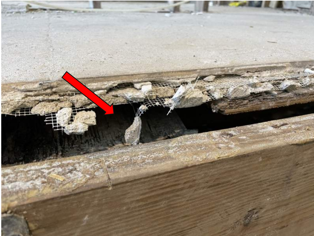
Photo 3 – Damaged or Failed Subfloor
