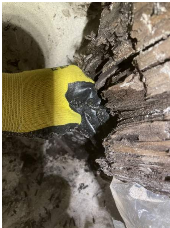
Photo 8 – Timber Pile Cross Section Loss
