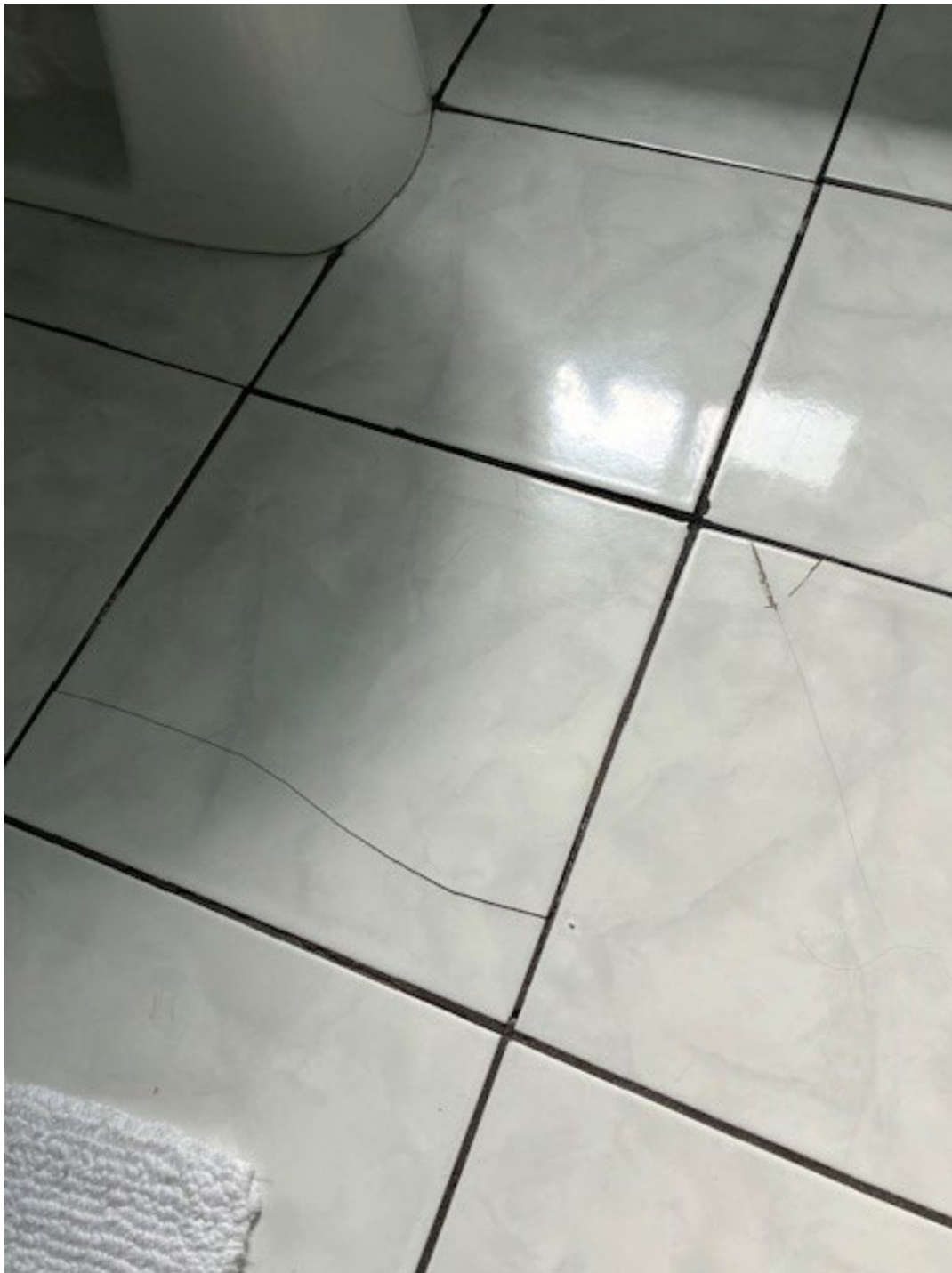
Floor/subfloor in bathroom near shower and toilet is soft and needs to be repaired. Broken floor tile needs to be replaced.
