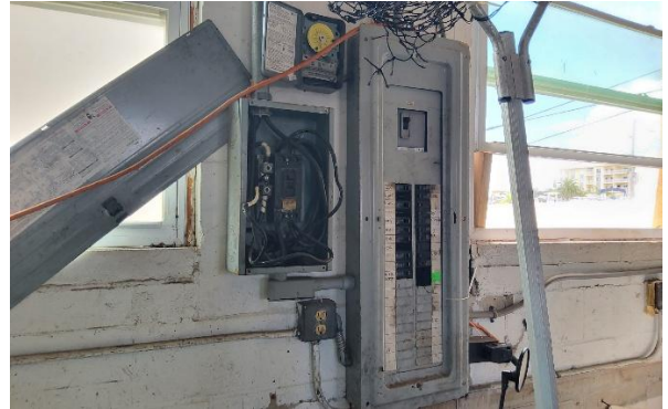
WORK AREA ELECTRICAL PANELS
