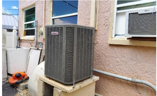
CENTRAL AIR COMPRESSOR 2ND FLOOR APARTMENT
