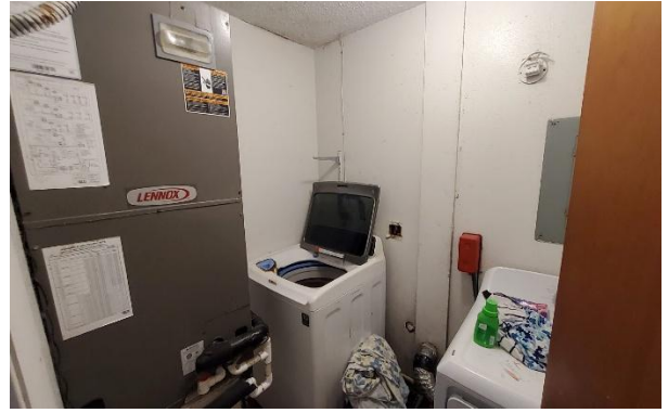
LAUNDRY AIR HANDLER
