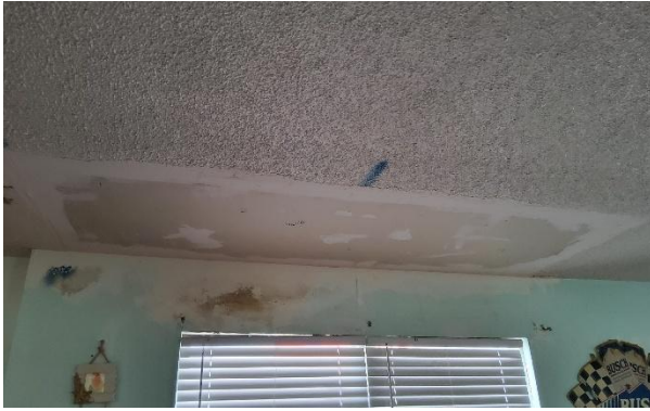
LIVING ROOM DEFERRED MAINTENANCE
