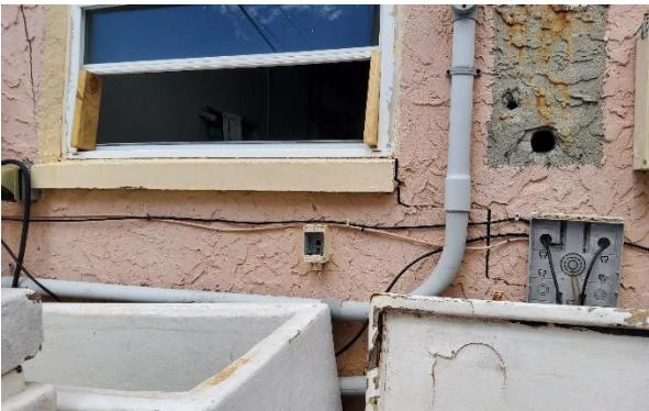
DEFERRED MAINTENANCE CRACKING STUCCO
