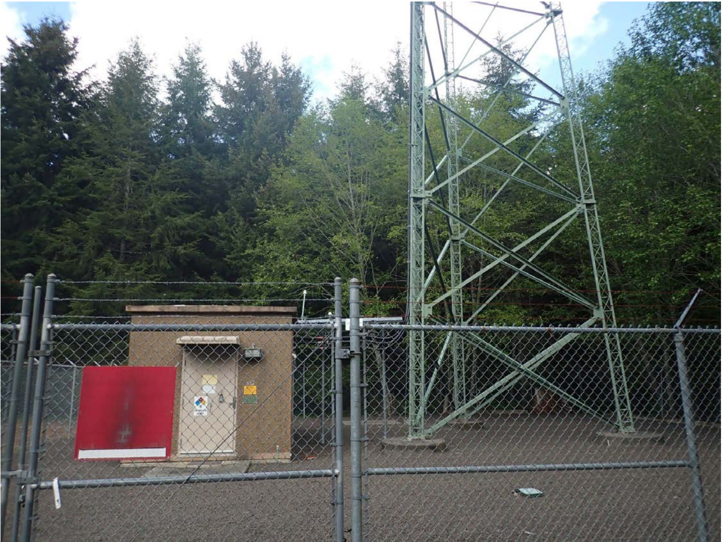
Image 10: Looking north at the comms shack and comms tower in the northeast corner of the fenced-in utility compound. The shack and tower are located within a second locked perimeter. PNSN will acquire keys for gate access.
