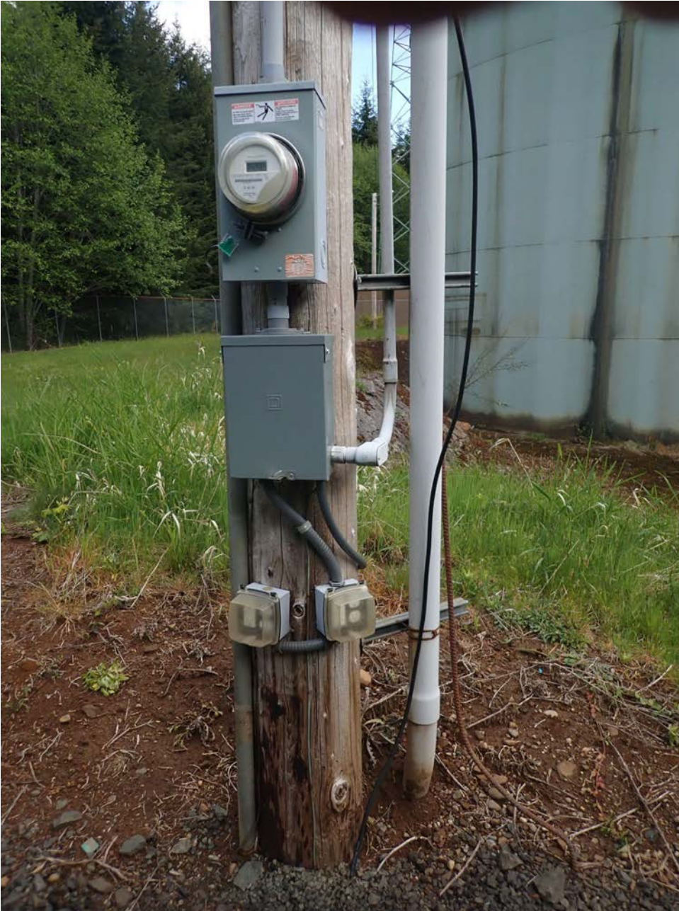
Image 9: Looking east northeast at the AC power pole that will provide power for the instrument. AC power will be converted to low voltage DC power and trenched to the post and power enclosure. The precise path of trenching will depend on the location of other buried utilities (fiber). A small repeater box will need to be mounted to the power pole to host the AC to DC power converter. An electrician will need to be onsite to pull power from the power pole.
