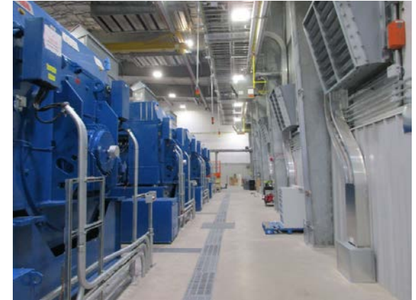
Westside Energy Station 5x9 MW
