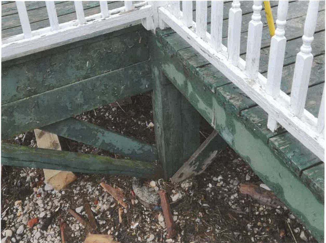
Photograph #2: View of the existing deck foundation. (Project No. 2022.2381, Thunderbird Gifts – Deck Settlement, Mackinac Island, January, 2023)
