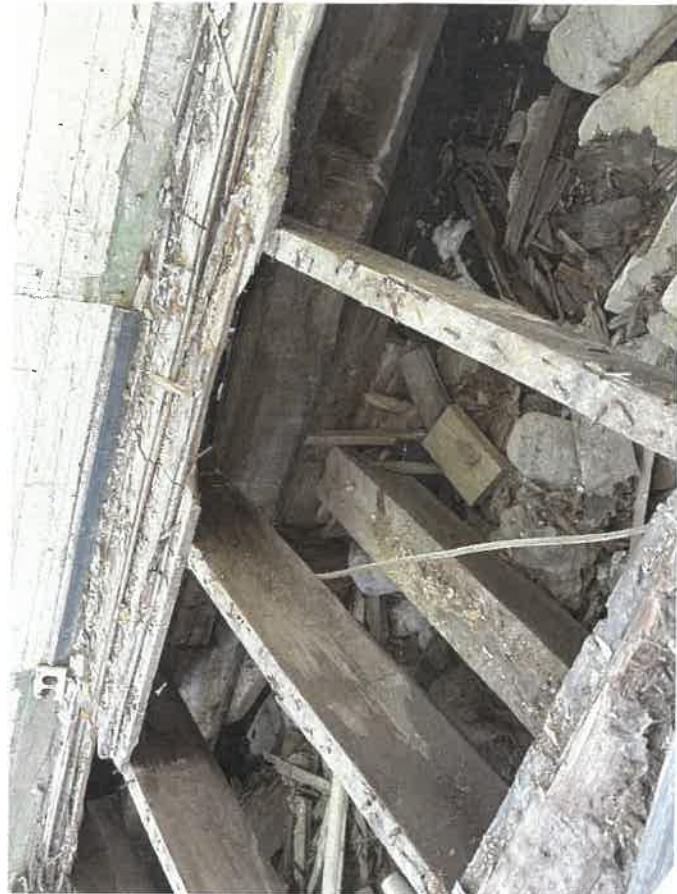
Foundation Obsolescence & Failure
