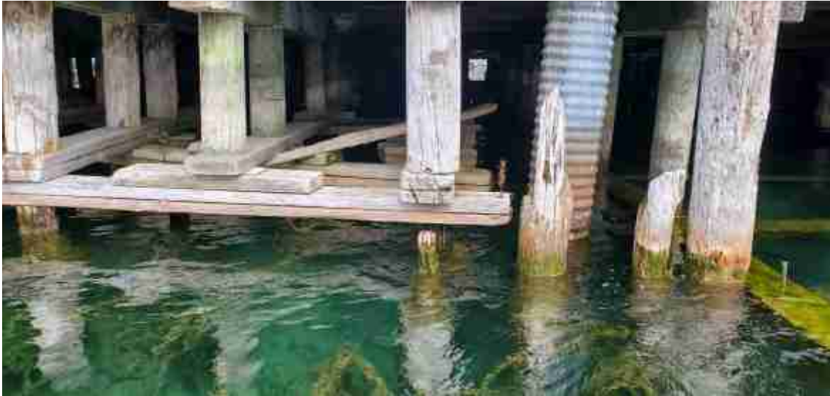
Excessive benching/missing or deteriorated piles
