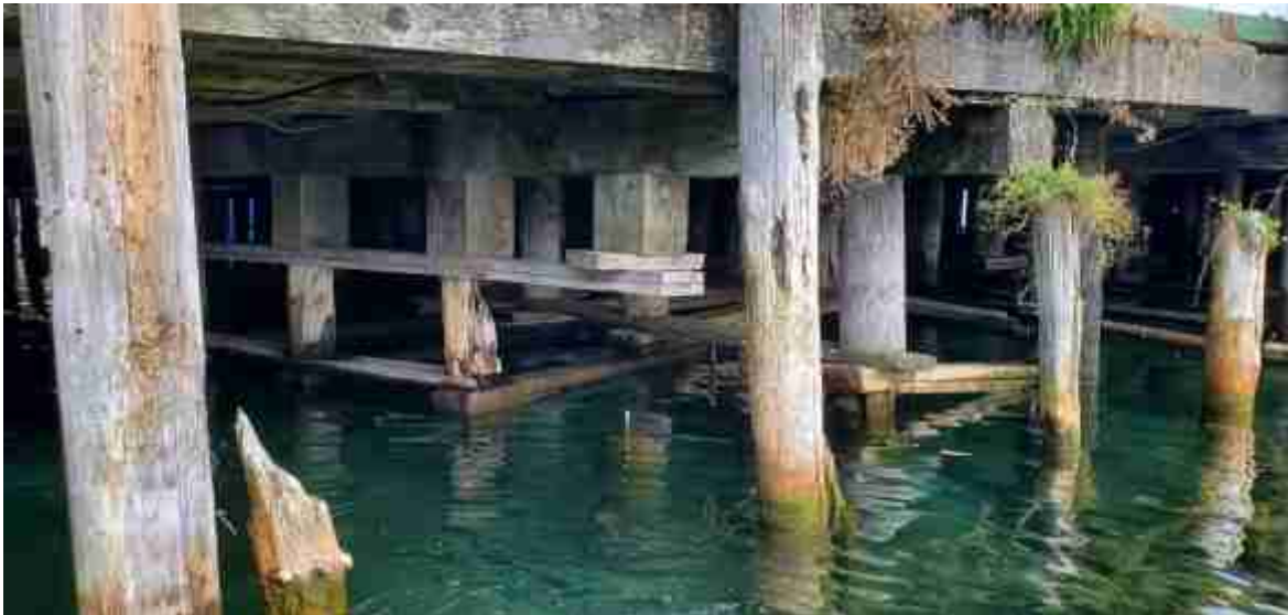
Excessive benching/missing or deteriorated piles
