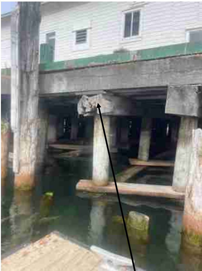
25) Dock (south) (west end) Main girder deterioration
