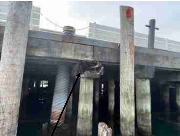
79) Dock (north) Deteriorated beam
