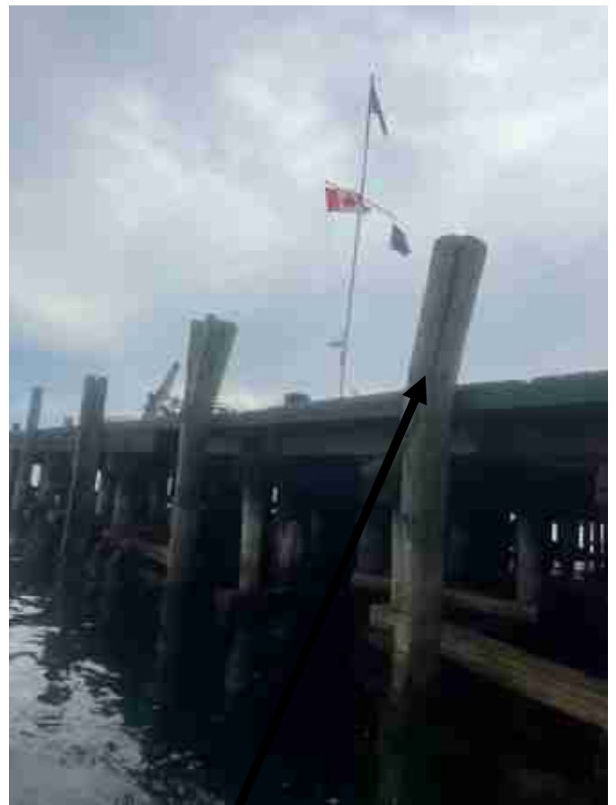
54) North side east end Bumper piles damaged
