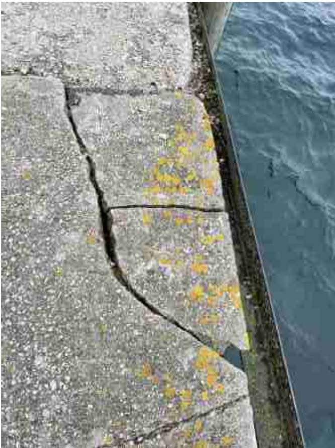
124) Broken deck, angle separation
