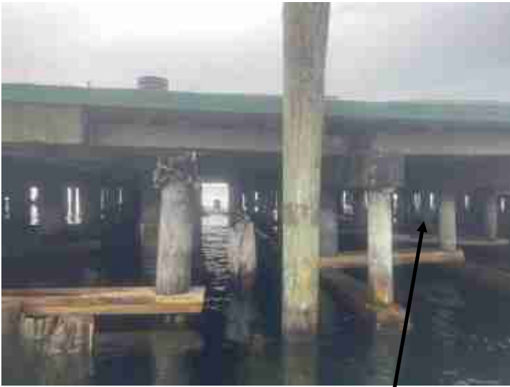
53) North side east end Excessive benching
