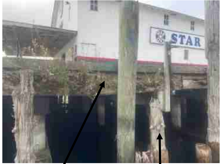
62) Dock (north) Deteriorated beam Deteriorated piles
