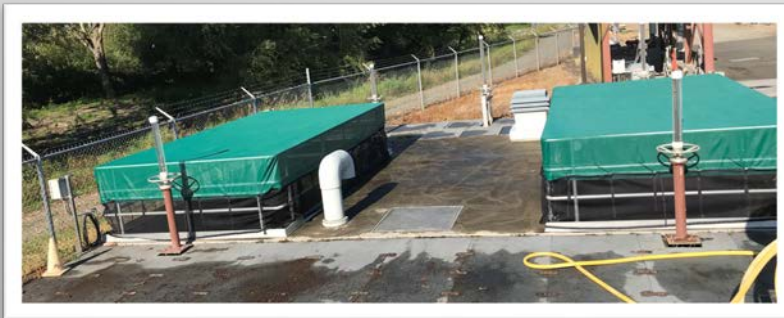
WWTP Effluent Filter Covers
