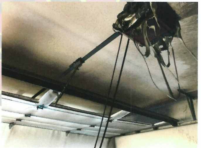
Bluestem garage fire
