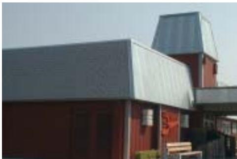
Unacceptable Hip on Deck Too Tall
