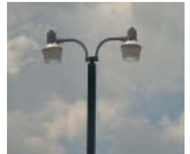
Unshielded lighting is distrubing to neighboring homes.
