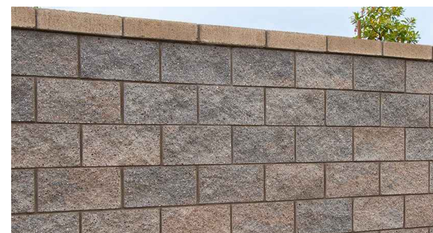
A RETAINING WALL SHALL BE VARIEGATED CMU WITH WALL CAP FROM ORCO BLOCK AND HARDSCAPE COLOR SHALL BE BORREGO SPLIT FACE ON EXPOSED SURFACE LRV SHALL BE MAX 30%
