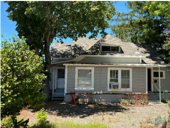
Image J. Rear Facing Shed Dormer Proposed For Removal
