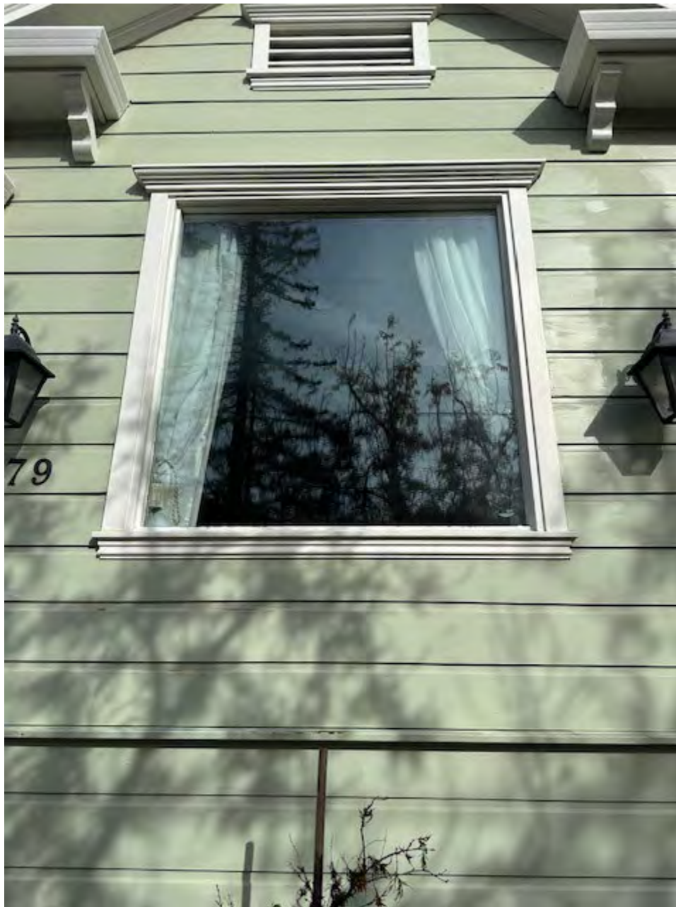
Window to be replaced
