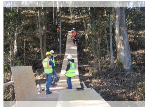
SWCA constructed a ramp to skid vegetation over a creek without heavy equipment.
