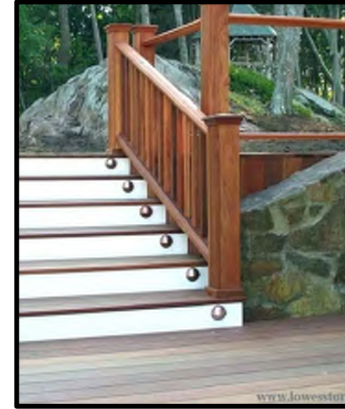
HANDRAIL AT STEPS
