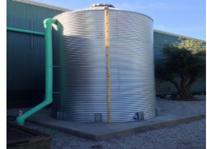
Figure 2-7 Rainwater Harvesting cistern, Environmental Innovation Center, San Jose (Source: City of San José)
