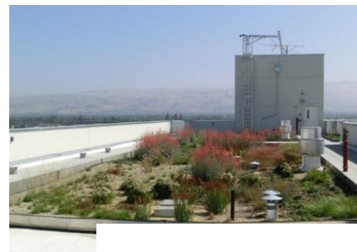
Figure 2-6 Green Roof at Fourth Street Apartments, San Jose (Source: EOA)
