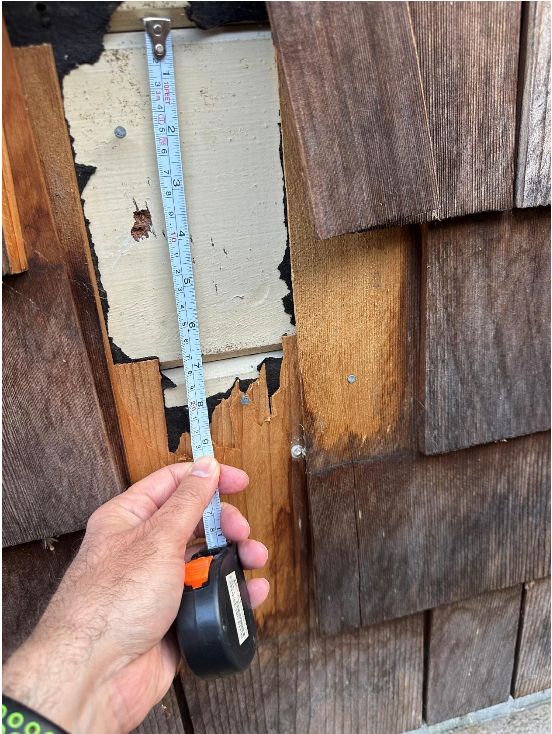
Old siding (allegedly): also 7"
