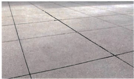
VEHICULAR COLORED SAWCUT CONCRETE PAVING COLOR: DARK GRAY BY DAVIS COLORS FINISH: MEDIUM BROOM FOR THE MAIN COURT; TOPOCAST 25 FOR THE INTERIM PARKING STALLS
