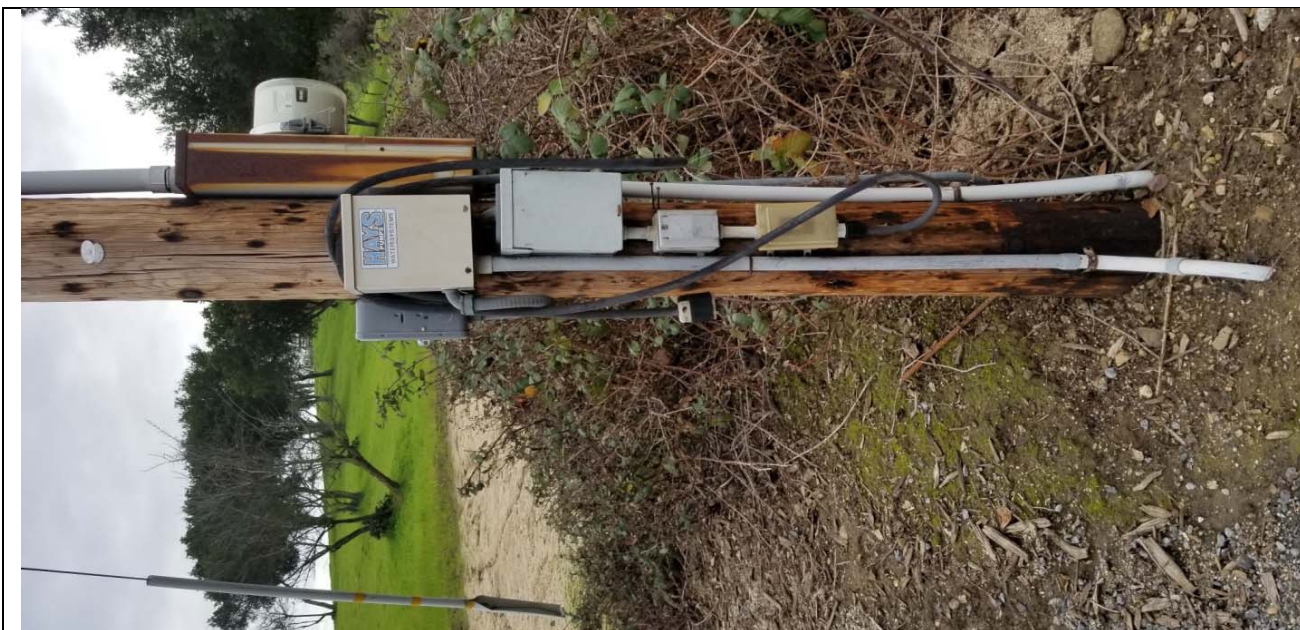
6. Power Pole at LOT 1
