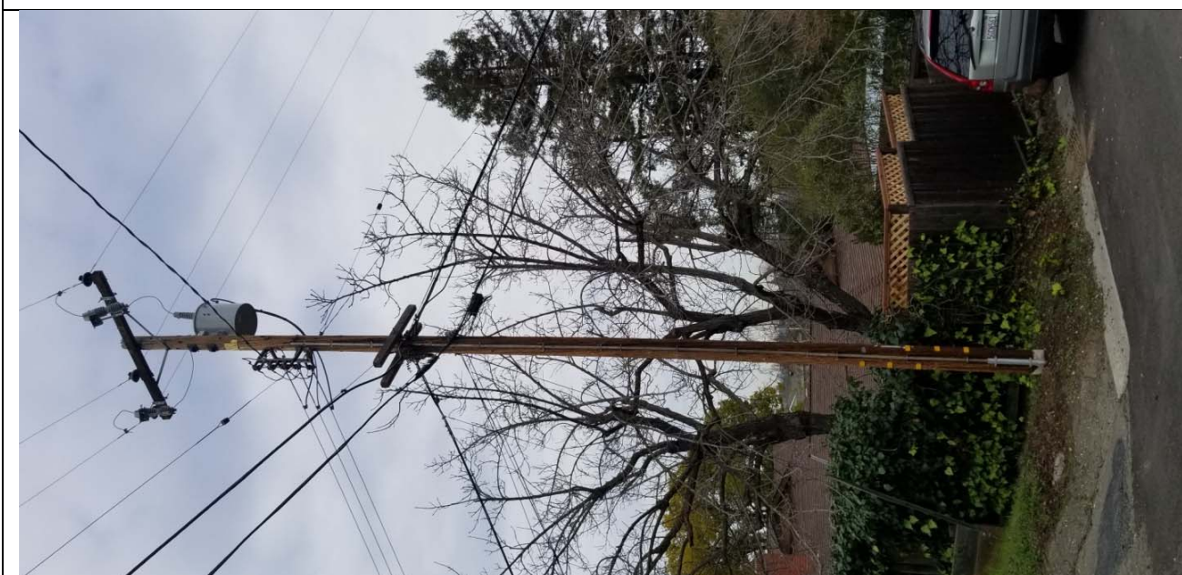
7. Power Pole at LOT 1
