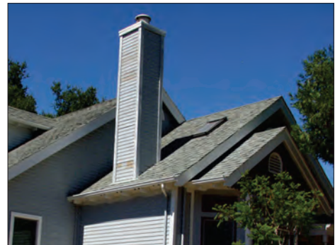
Wood clad chimneys are prohibited
