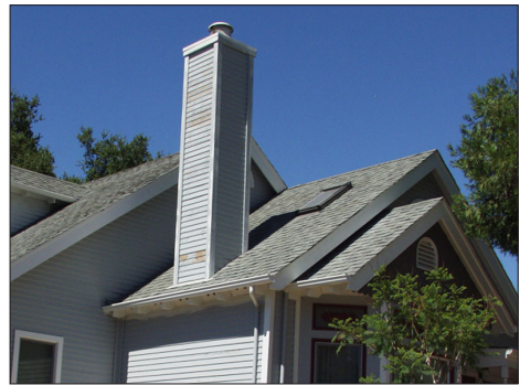
Wood clad chimneys are prohibited
