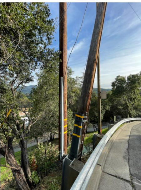
Severely leaning powerline. (Hillside burned in 1997 due to PG&E fire).
