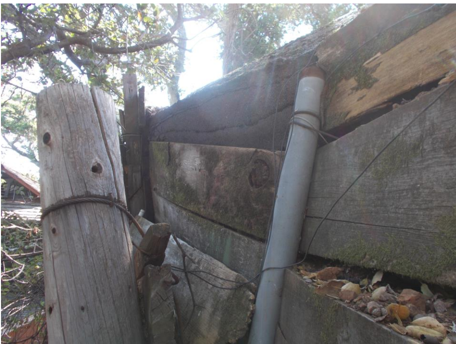
Photo 8 – Photo showing various repairs. Paving at parking now exposed as lagging has slid down.
