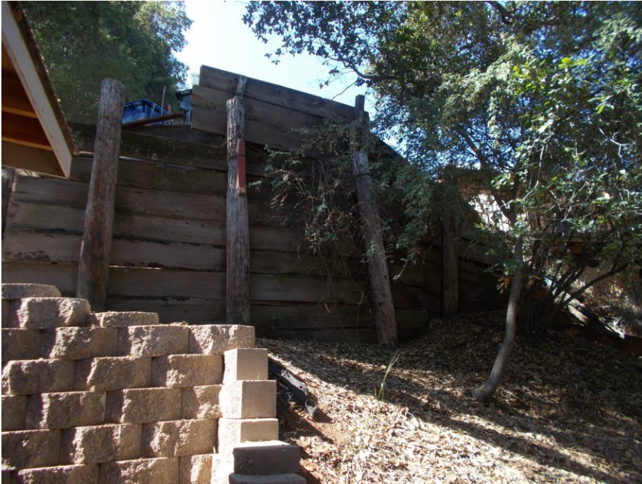
Photo 1 – Over view of retaining wall. Note proximity of roof overhang of residential init.
