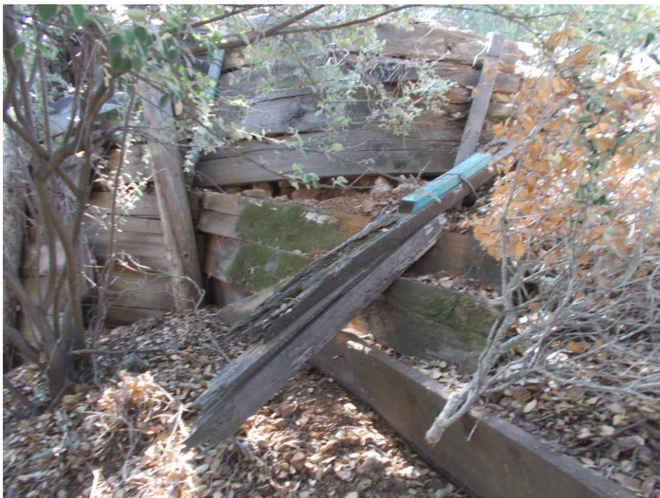
Photo 10 - Wall failure from degradation of components at right (East) end of wall. Excessive deflection of lagging in upper wall is another potential failure mode.
