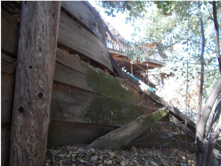
Photo 9 – Wall failure from degradation of components at right (East) end of wall.
