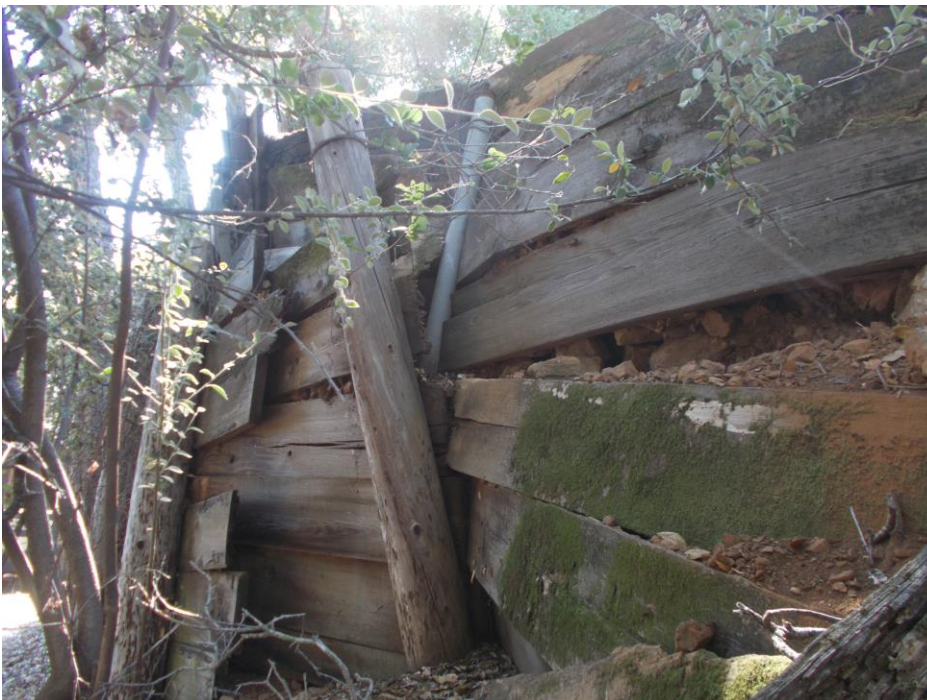
Photo 6 – Leaning column where cable holding top of column failed.
