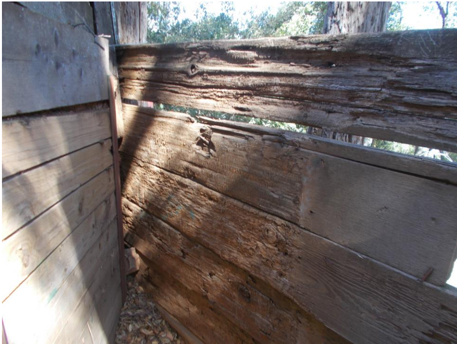
Photo 3 – Dry rot visible on back of lagging. Amount varies by location.
