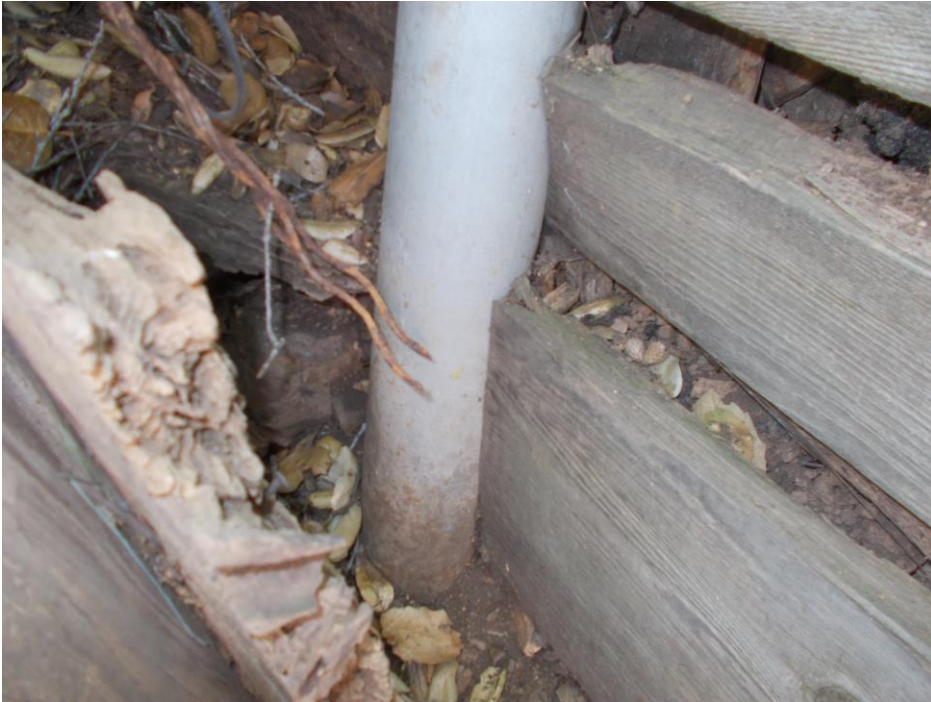
Photo 7 – Rusted end of cable where it failed and pulled out of soil. Inadequate bearing of lagging at steel column repair.
