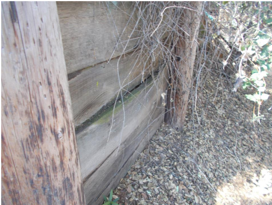
Photo 4 – Excessive deflection of lagging.
