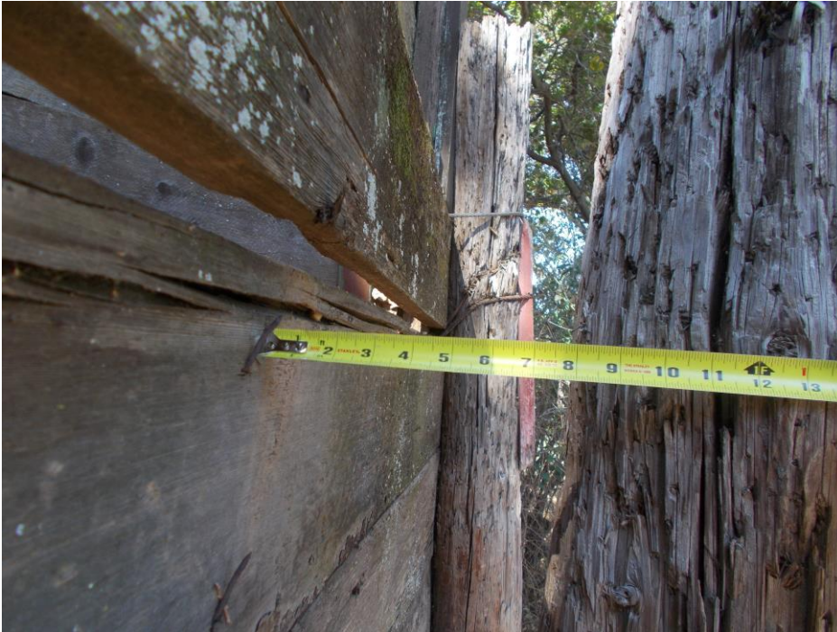
Photo 5 – 8" space between lagging and displaced column.
