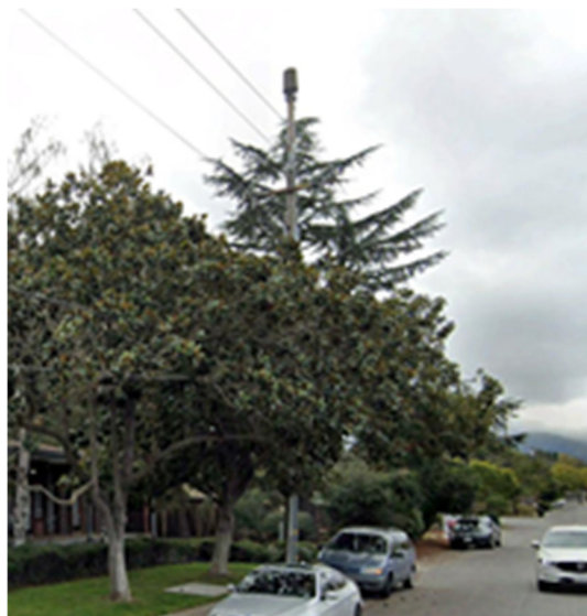
Figure 7: Landscaping conceals wireless telecommunications equipment mounted on the exterior of this pole located on Distel Drive.
