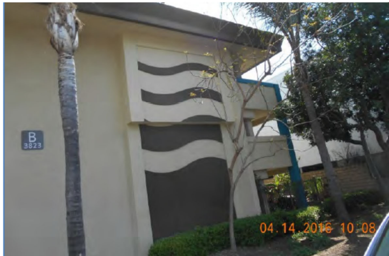
Figure 5: Although façade-mounted boxes are not preferred, this example from San Diego achieves integration with the structure.
