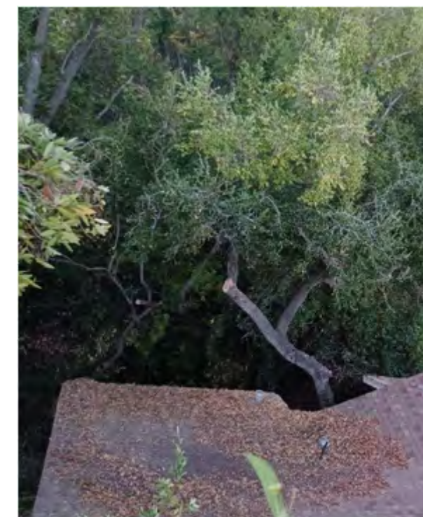
Clearance to Cottage (Tree 7, 8)
