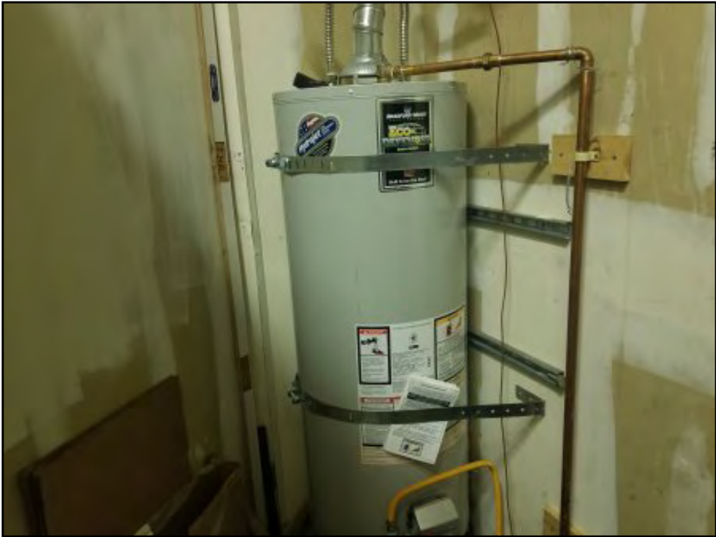
19 : View of the water heater for the building.
