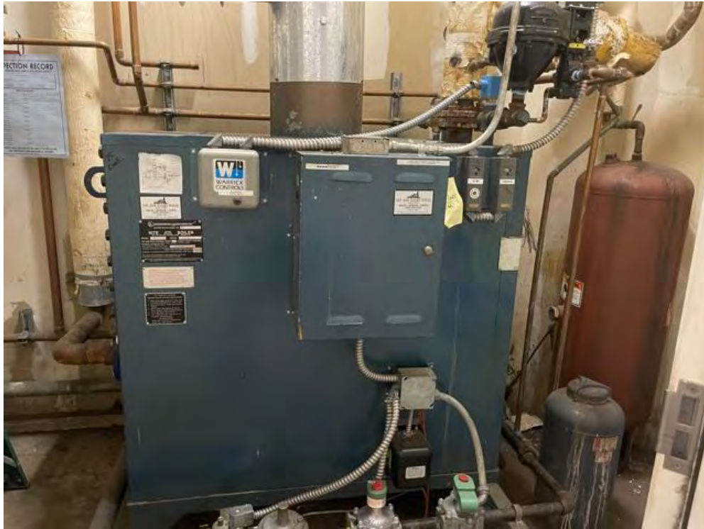
PHOTO #9. VIEW OF BOILER ROOM.
