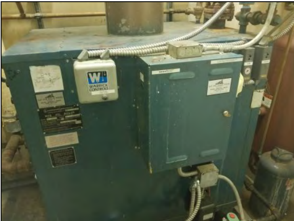
18 : View of the hot-water boiler for the building.
