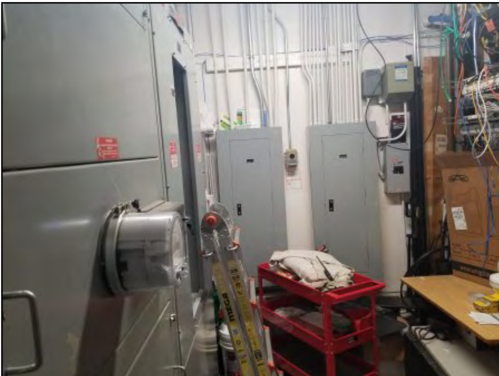
16 : View of the electrical room.
