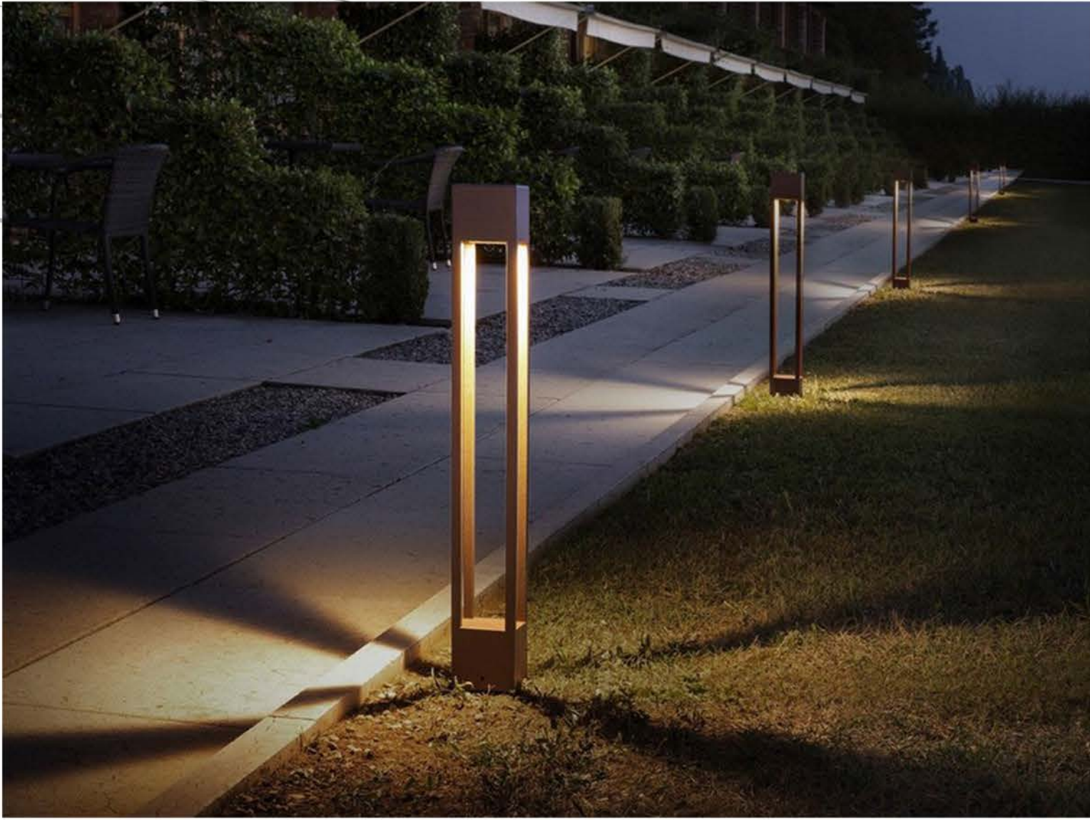
+ ENTRY AND COURTYARD BOLLARD LIGHTS
