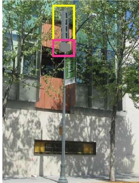
Figure 8: Stand-alone small cell poles (as shown in this example) are not preferred but may be permitted if enclosure of all equipment within the pole or in an underground vault is technically infeasible.
