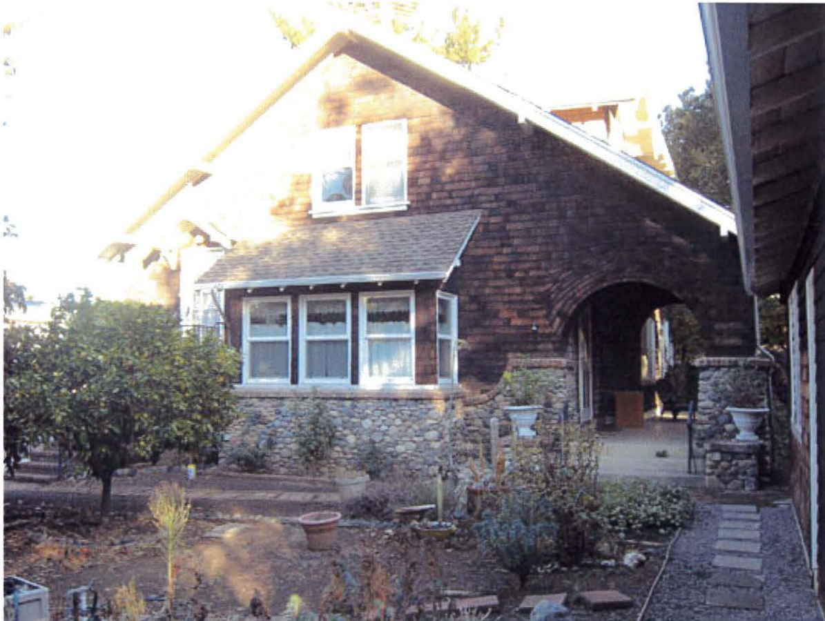
View of the east/front elevation of the house. Work to the first floor windows is not included in this phase. Work to the second floor windows is discussed below.
