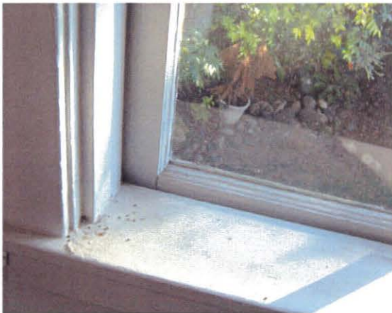
Image showing warped casement sash in the western grouping of casement windows at this elevation.
