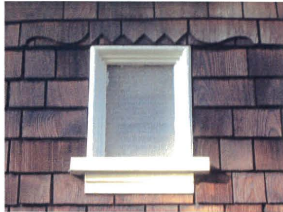
The above window is proposed for removal. It faces the east side garden and is not visible from a public right-of-way.
