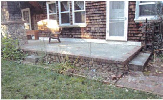
View of the existing patio proposed for removal and replacement with a larger concrete patio. Given that the patio is screened from public view by the side porch, the new patio will not be visible from Grant Road.
