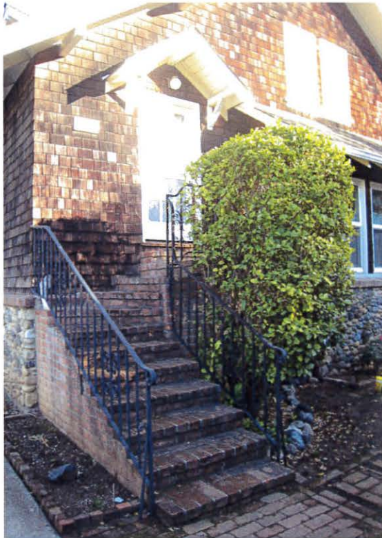
View of the brick exterior stair at the south side of the east elevation.
