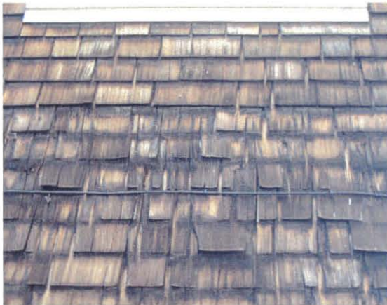
View of wood shingle damage at the south side of the west wall, between the first and second story windows. Damaged shingles will be replaced with cedar shingles. Less than 10% of the shingles need replacement. Transparent shingles stains will be tested to determine if staining will blend the new with the old; if successful, the new shingles will be stained to blend new shingles with the adjacent old shingles.
