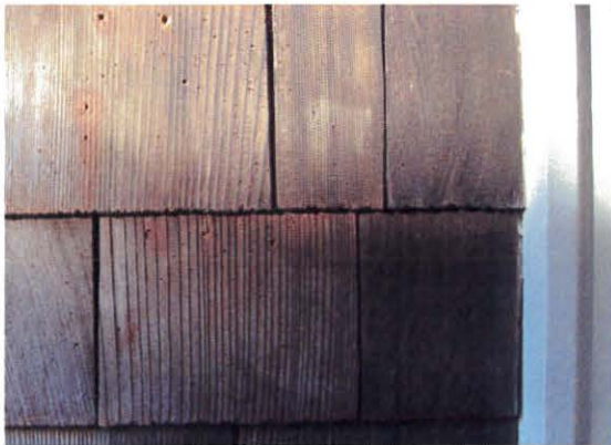
Detail view of north porch shingles which appear to be sawn redwood. These shingles are probably original to the building.
