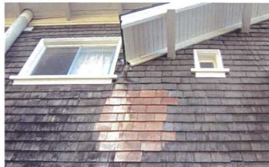
The windows at the left are non-historic sash which will be replaced with double-glazed, wood casement sash with interior and exterior grids to suggest the same light configuration as the adjacent historic windows. The small window at the right is the third and final small window proposed for removal.
