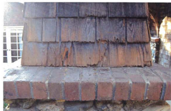
View of wood shingle damage at the north porch.
