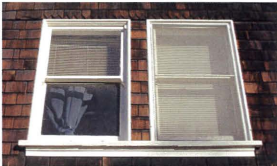
View of the second floor windows at the east elevation. These windows are wood one-over-one light, double hung sash in good condition. The windows will remain, but they will be re-glazed with laminated glass without a tint.
