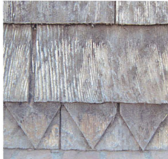
View of wood shingle deterioration due to the loss of lignin, probably caused by ultra-violet light.
