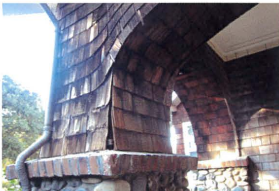
View of wood shingle damage at the north porch.
