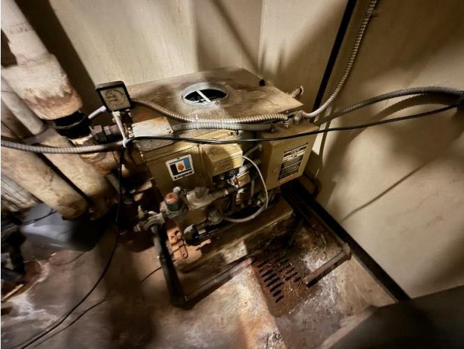
61. Decommissioned water boiler
