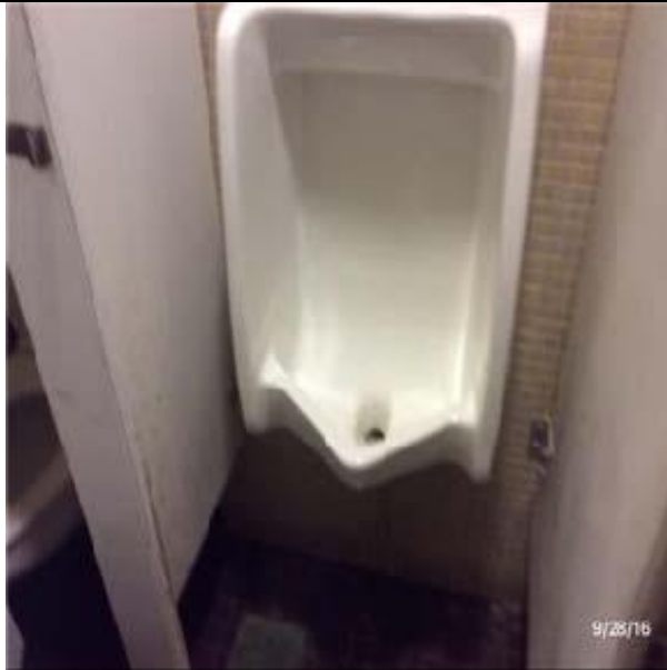
D2012 Urinals:- View of Wall Hung Urinals
