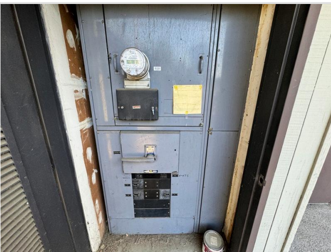
47. Main electric distribution panel
