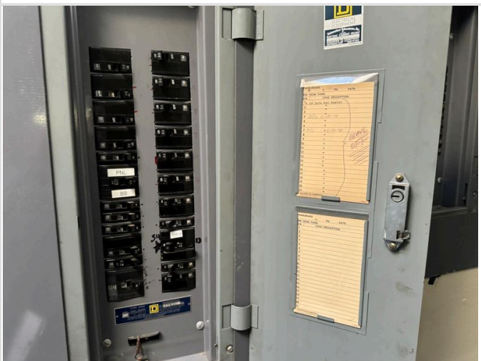
48. Electric breaker panel
