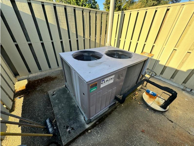
49. Grade-mounted HVAC unit
