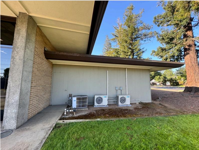
51. Ground mounted HVAC unit
