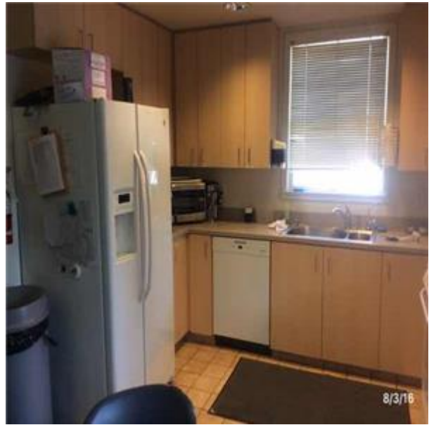
E2012 Fixed Casework:- View of Floor Mounted Base Cabinet(s) - Standard
