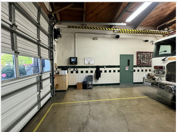
42. Garage interior, cracks observed on the flooring
