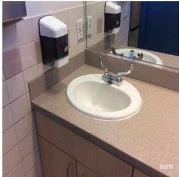
D2013 Lavatories:- View of Vanity Top Lavatories
