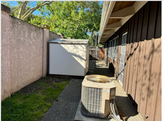
34. Grade-mounted HVAC unit
