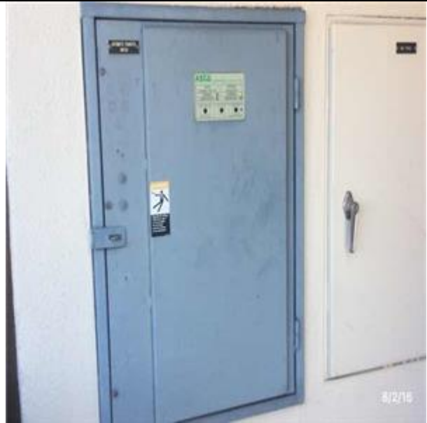
D5012 Low Tension Service & Dist:- View of Emergency Generator Transfer Switch
