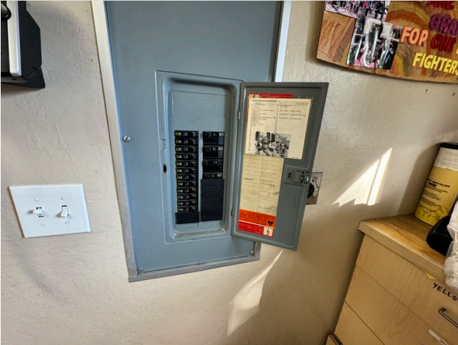
31. Electric breaker panel
