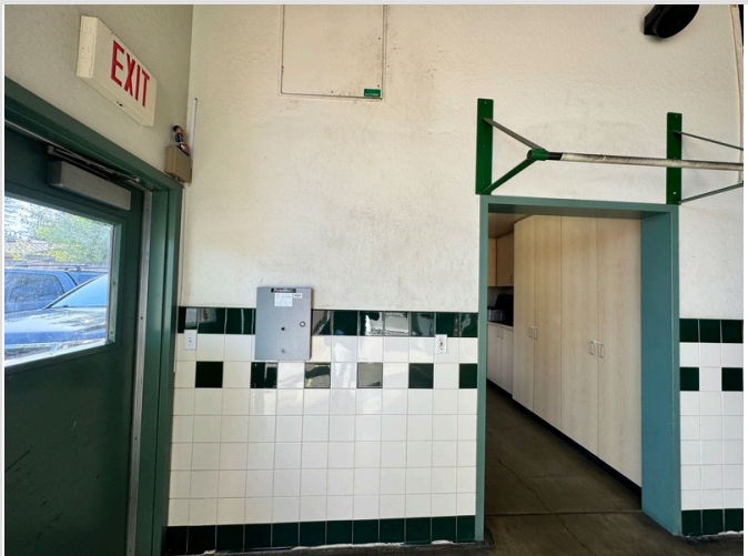
40. Illuminated exit sign
