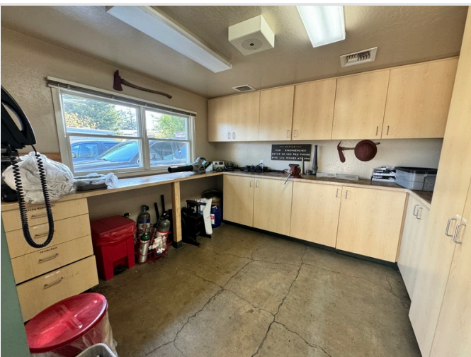
41. Cracks observed on the flooring
