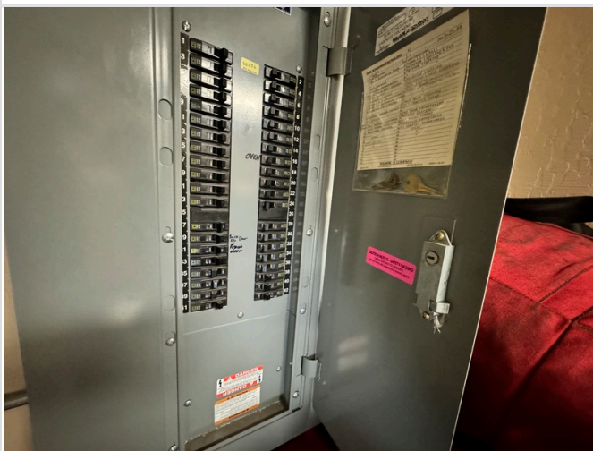
30. Electric breaker panel
