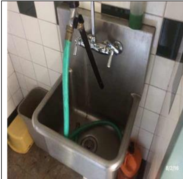
D2014 Sinks:- View of Service Sink Wall Mounted
