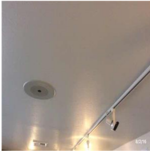
D5022 Lighting Equipment:- View of Track Lighting Fixtures
