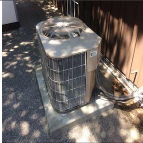
D3032 Direct Expansion Systems:- View of Split-System (Outdoor Unit Only - Compressor and Condenser)
