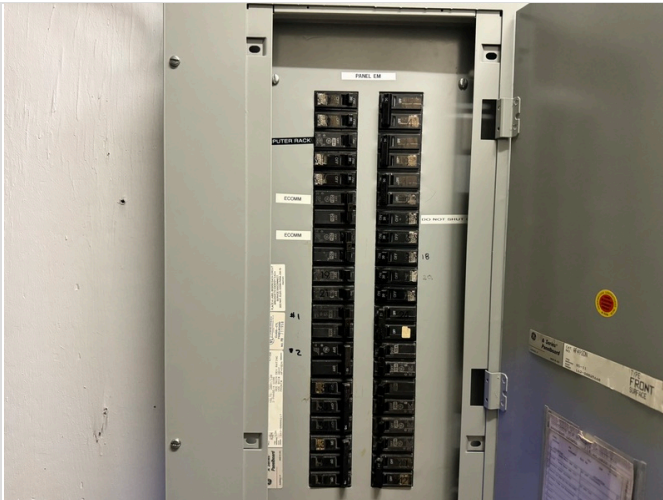
38. Electric breaker panel
