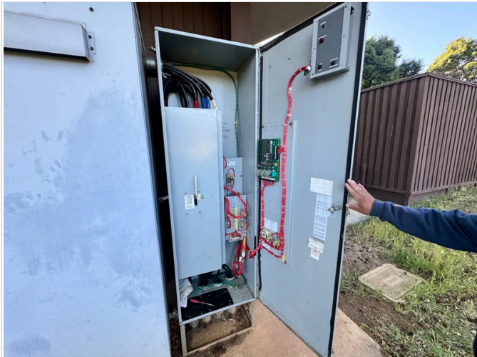
37. Electric breaker panel
