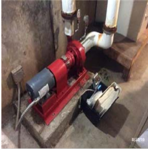
D3044 Hot Water Distribution:- View of HW Circulation Pump/Motor 1-2 HP
