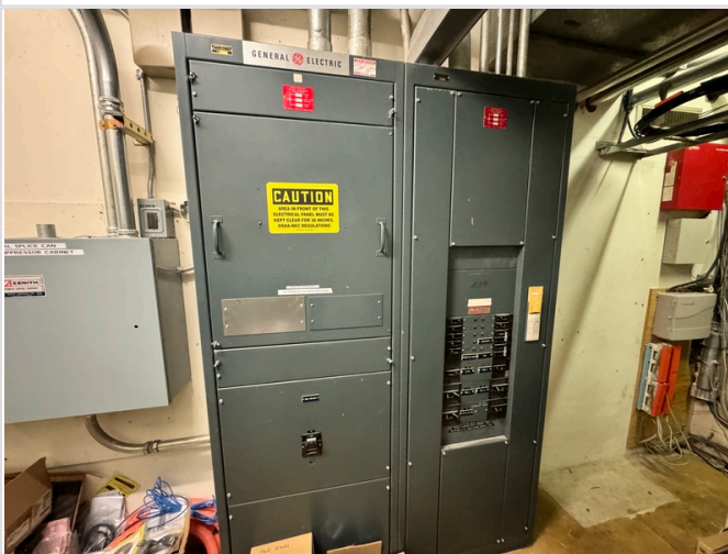
36. Main distribution panel
