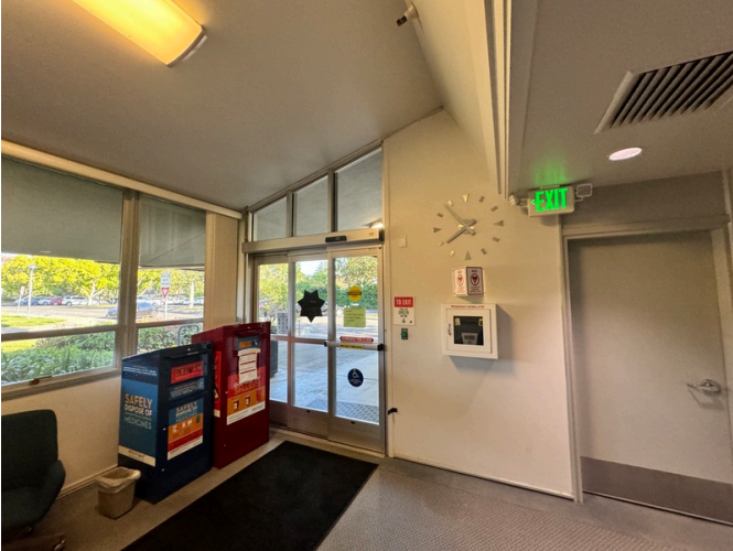
43. Illuminated exit sign
