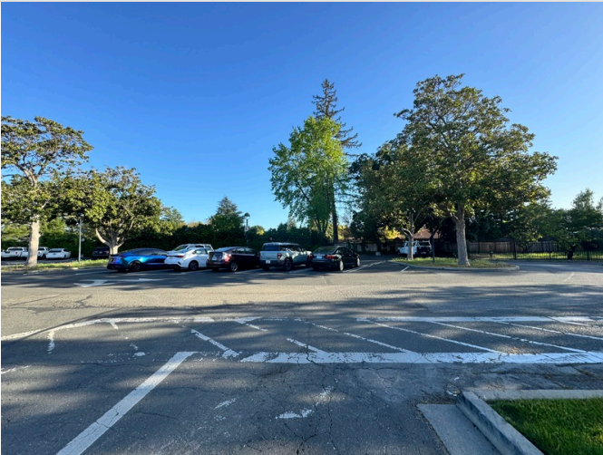
45. Cracks and alligating observed on the pavement
