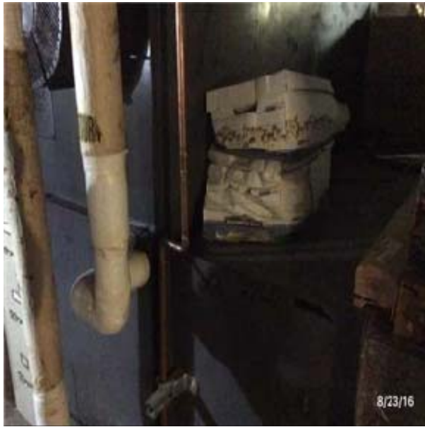
D3041 Air Distribution Systems:- View of AHU - Constant Volume #1
