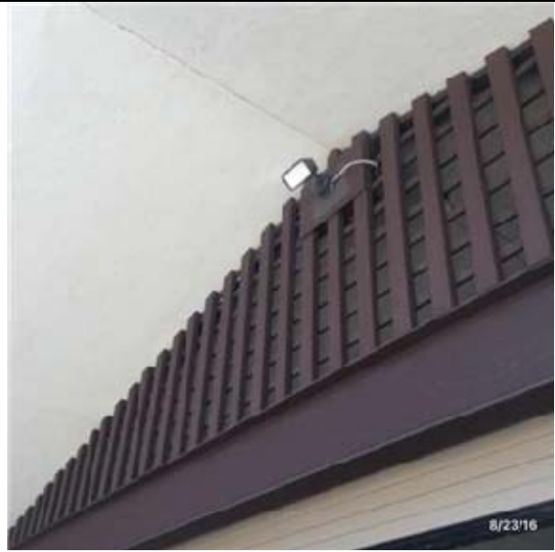
D5022 Lighting Equipment:- View of Flood Lights - Metal Halide Fixtures
