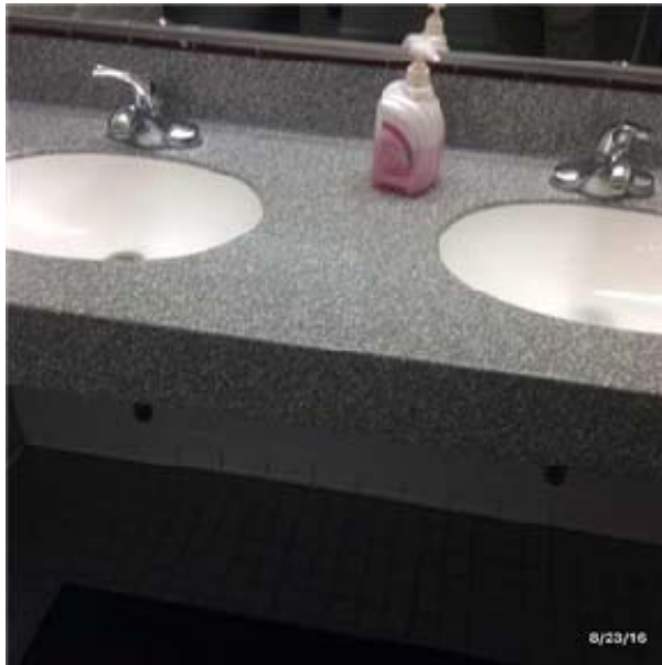
D2013 Lavatories:- View of Vanity Top Lavatories
