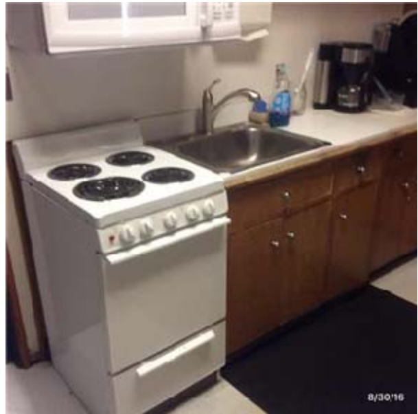
D2014 Sinks:- View of Single Bowl Kitchen Sink
