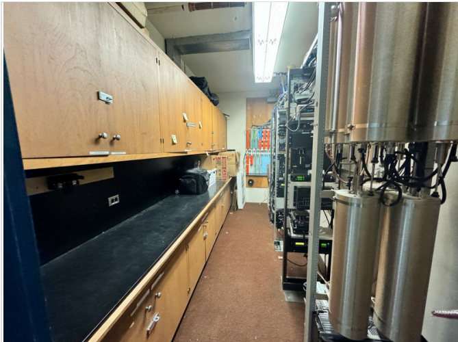
31. Mechanical room interior
