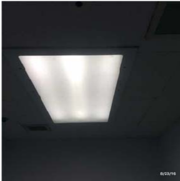
D5022 Lighting Equipment:- View of Interior Fluorescent Light Fixtures
