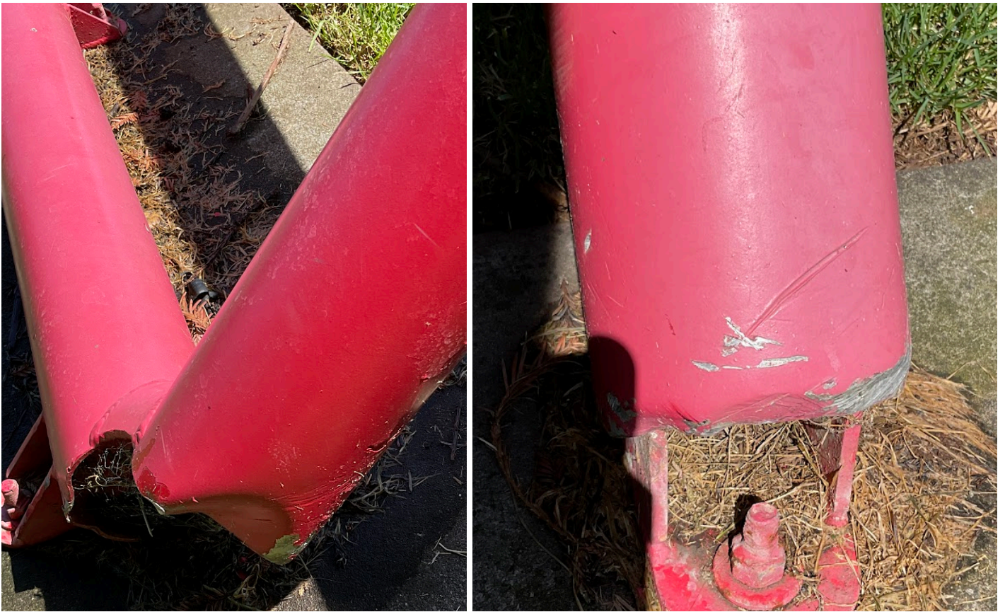
Details Showing Dents and Abrasions on the Bottom of the Lower Tubes
