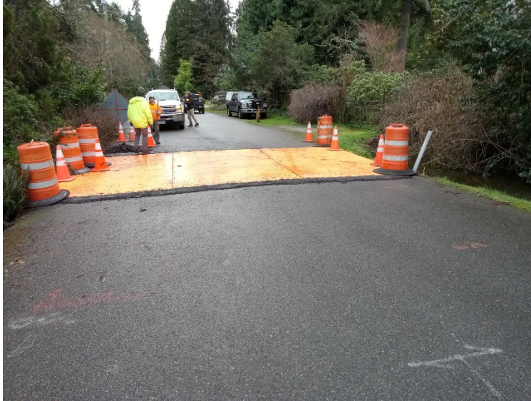
Photo: PW crew members and vendor staff complete installation of steel roadway plates
