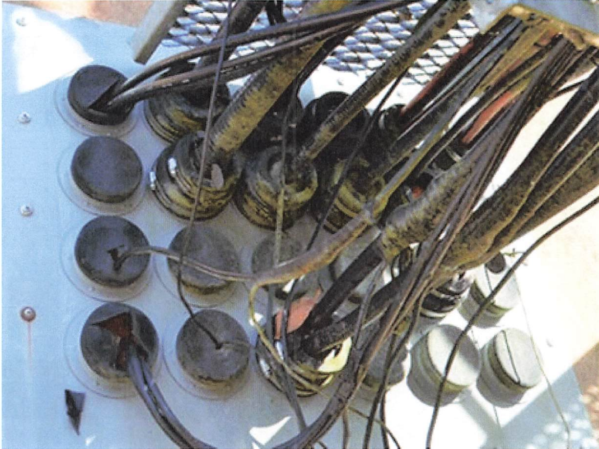
Figure 3 – Cable Entry Port
