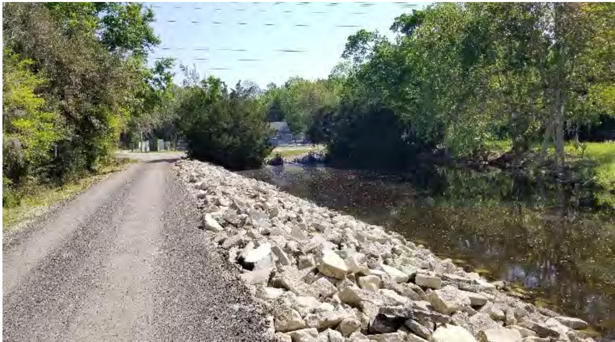
FIGURE 2: Sawgrass Pump Stations serve as critical assets to control flooding and provide community resilience.
