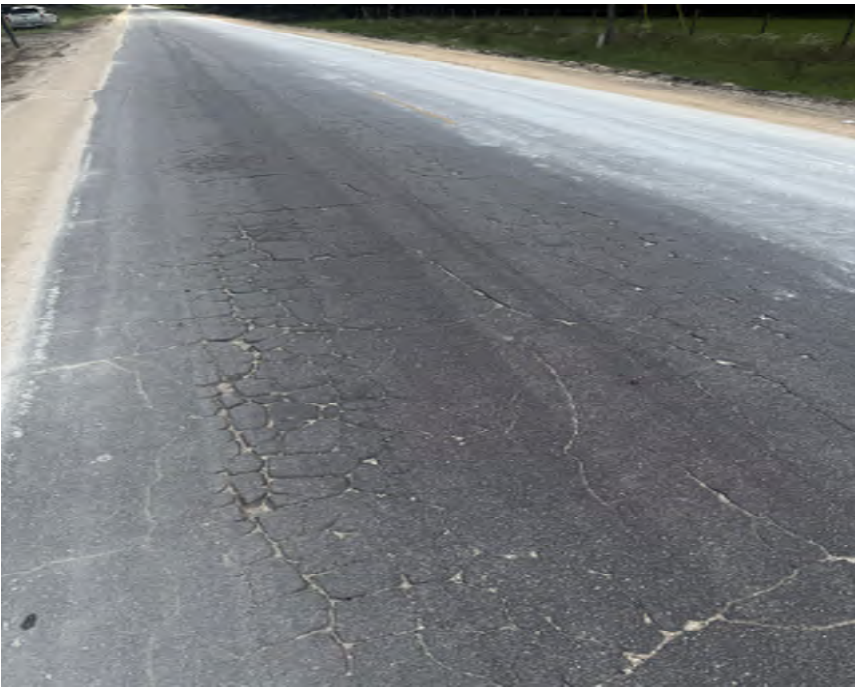
1374+00-1376+00 Asphalt cracking Thin Asphalt
