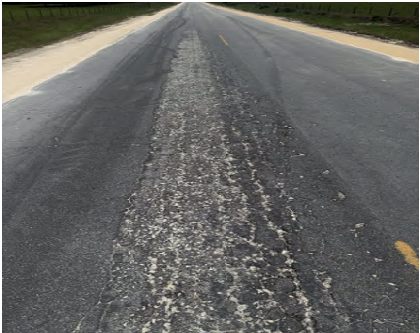
1326+00-1353+00 Asphalt cracking Thin Asphalt
