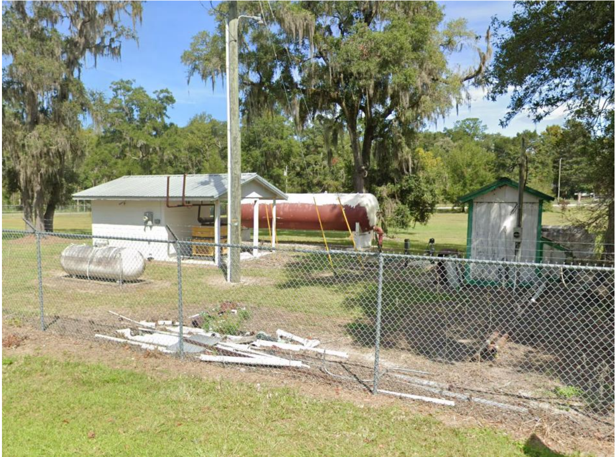
Figure 6: University Oaks WTP looking to the North
