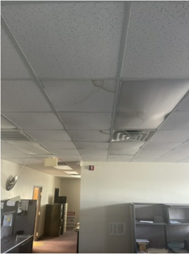
Interior View - Ceiling Damage
