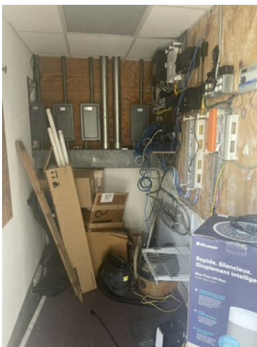
Interior View - Electrical
