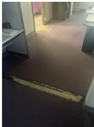
Interior View - Floor Damage
