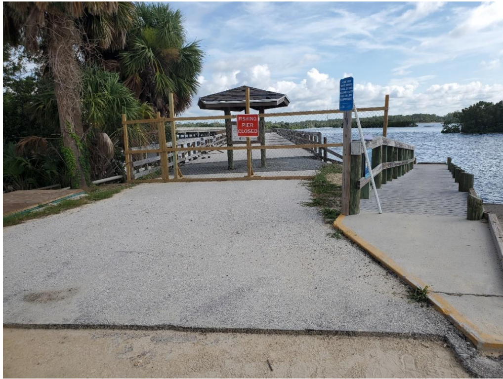
Photo 1: View looking north at asphalt approach of fishing pier. Pier closed.
