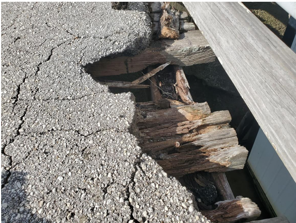
Photo 6: Deteriorated timber deck and failed asphalt overlay.
