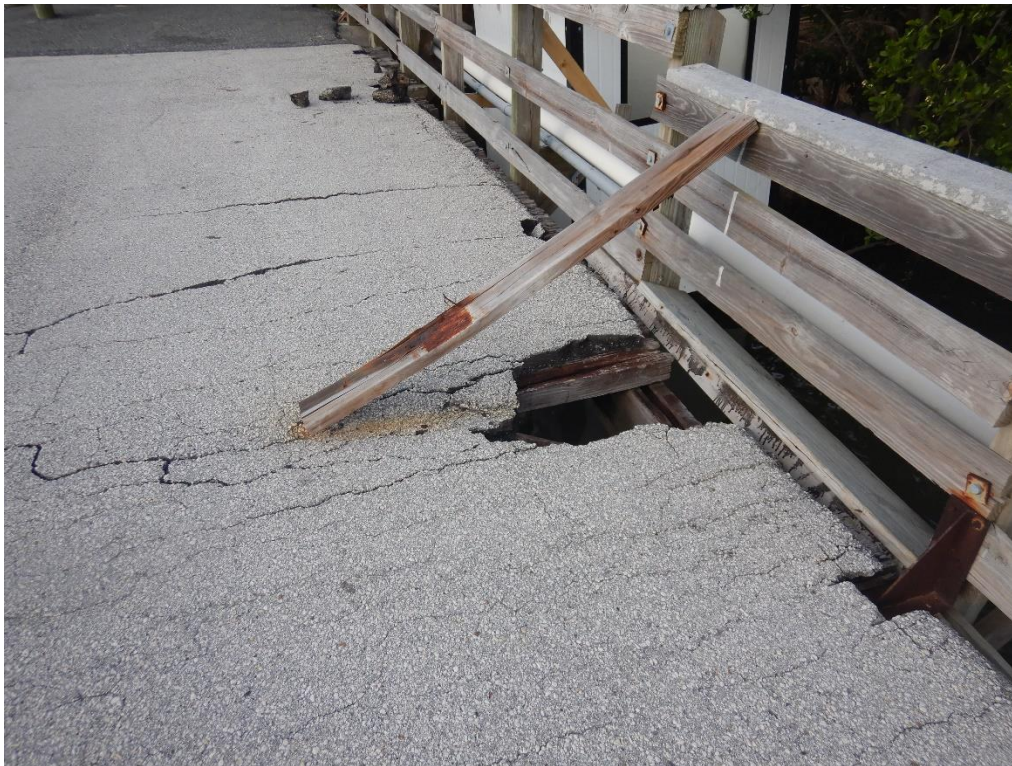
Photo 4: Failed timber deck and asphalt overlay. Note steel bracket supporting stanchion at bottom right.
