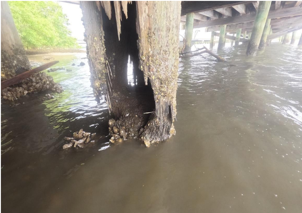
Photo 22: Pile 2C exhibiting significant loss of section due to marine borer attack. Pile is original.
