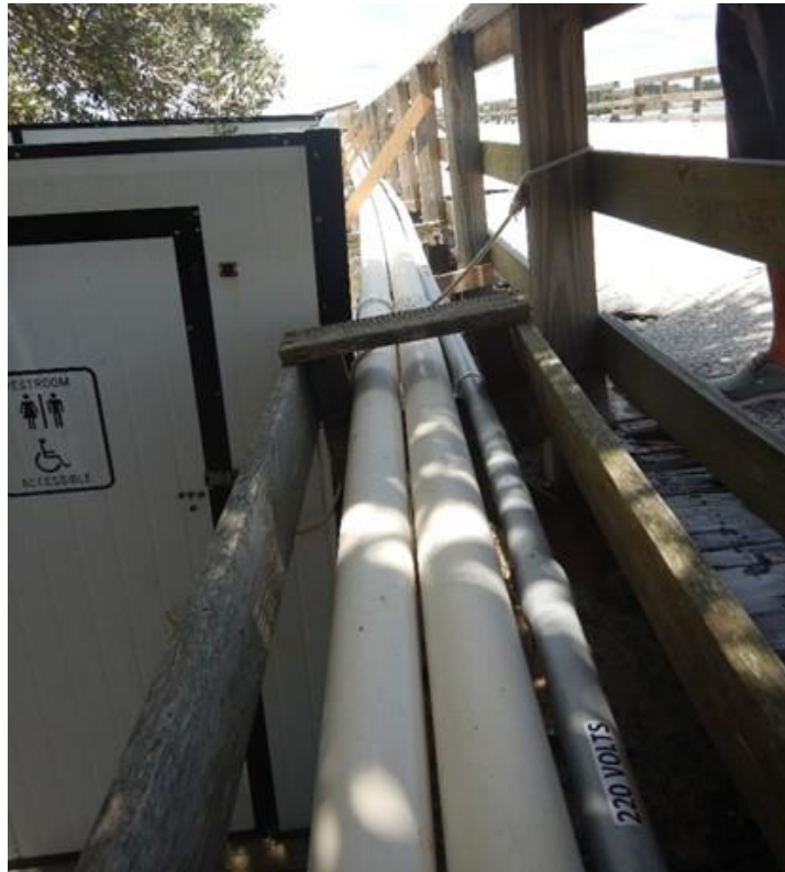
Photo 9: Three conduit secured to outboard side of western rail. Gray conduit on right labeled as “220 Volts”.
