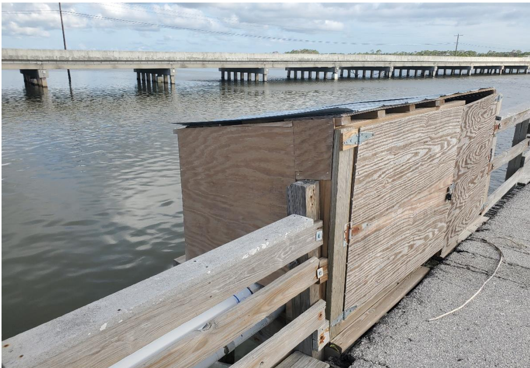
Photo 10: Pump enclosure at Bent 7 where conduits terminate.
