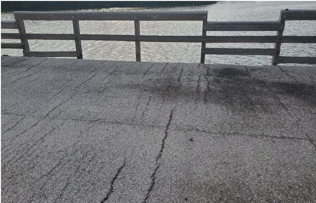
Photo 3: View looking east. Note transverse cracks in asphalt overlay and lowered rail sections.
