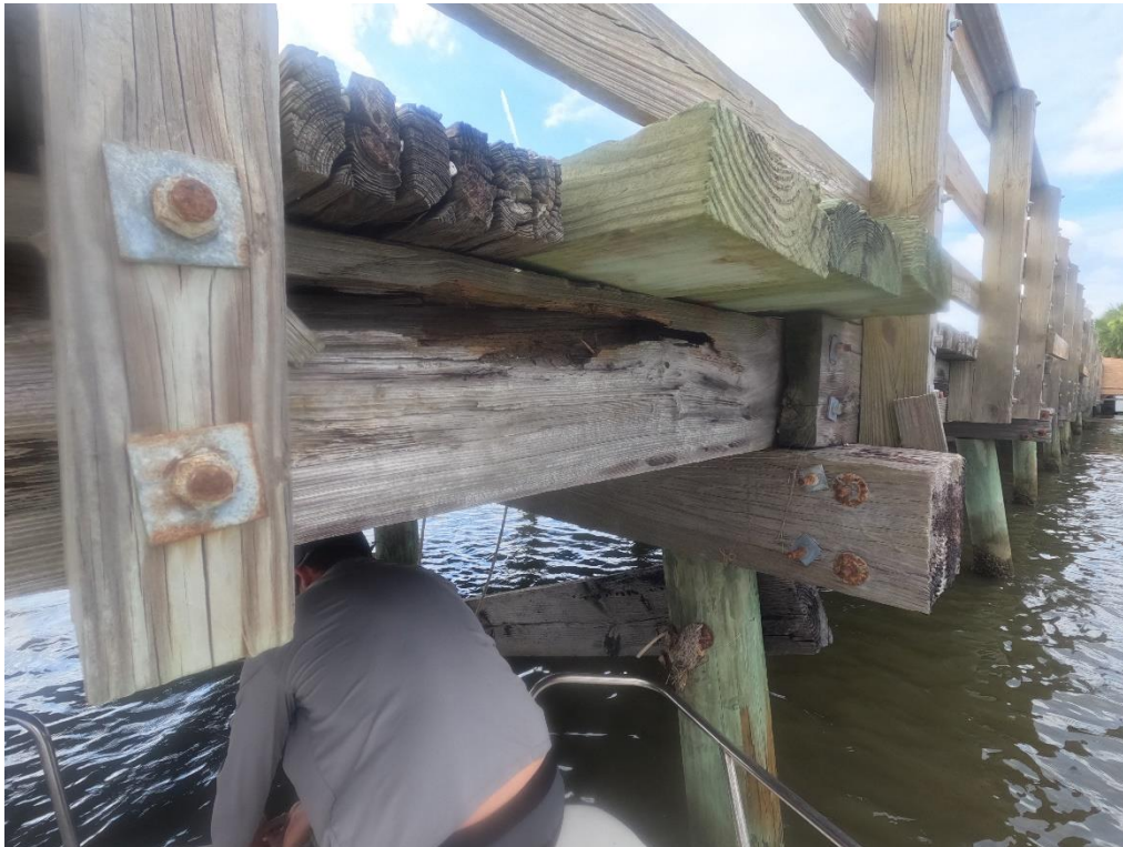
Photo 12: Bent 14. View comparing original 2 x 4 timber decking and CCA treated 4 x 12 members. Note large void in stringer from fungal decay.
