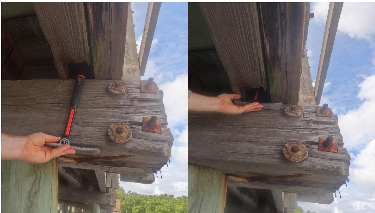
Photo 14 (L) and 15 (R): Void at end of stringer resulting from deterioration accommodating 10-inch inspection hammer handle.
