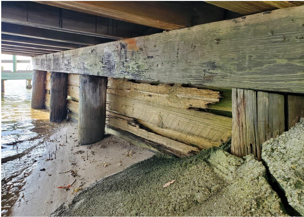
Photo 25: View looking east at backwall. Note multiple layers of timber and the outboard timber exhibiting loss of section caused by marine borer attack.
