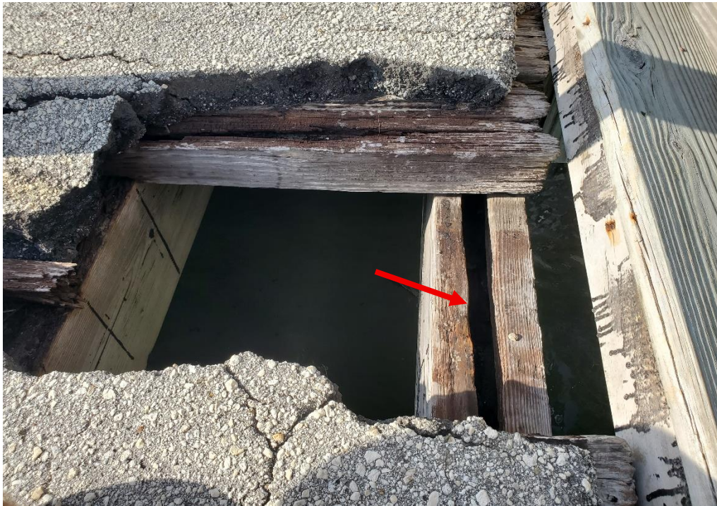
Photo 5: Deteriorated timber deck and failed asphalt overlay. Note void in center of 6x12 stinger (right). Moisture accessed interior heartwood through fasteners securing timber decking to stinger.
