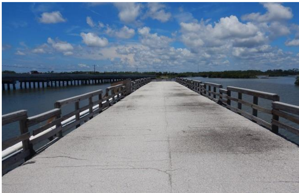
Photo 2: View looking north. Note transverse cracks in asphalt overlay and lowered rail sections.
