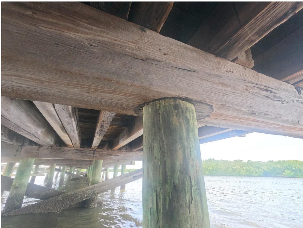
Photo 17: Underside of pile caps typically had dark circular stain indicative of creosote from original pile suggesting that the pile cap is original.
