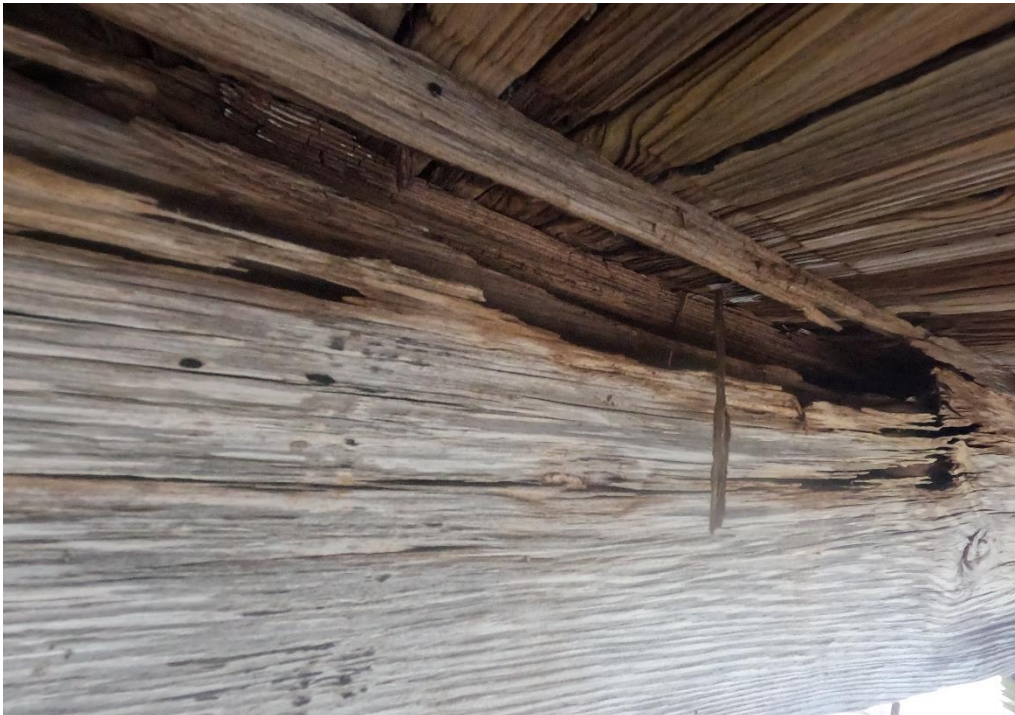
Photo 21: Significant void within stringer resulting from fungal decay.
