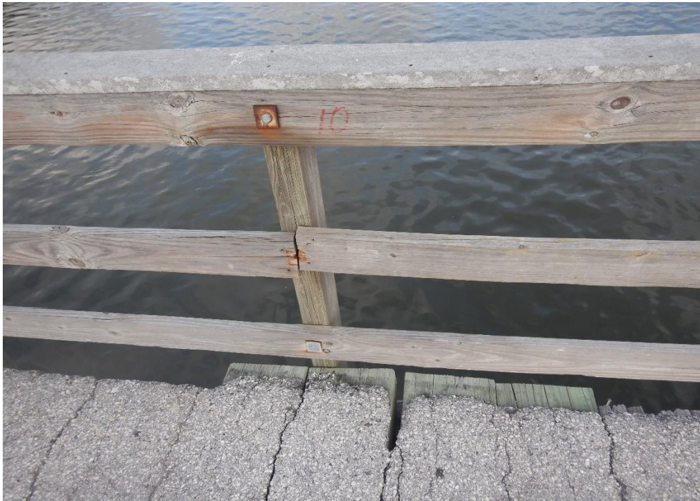
Photo 11: Bent 10. Original timber decking removed and replaced with four CCA treated 4 x 12 members when piles were replaced. Note transverse cracks in asphalt overlay.
