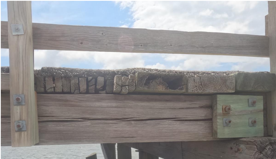
Photo 16: Original 2 x 4 timber decking exhibiting significant checks and shakes. CCA treated 4 x 12 exhibiting significant void due to fungal decay. Note longitudinal check in face of stringer.
