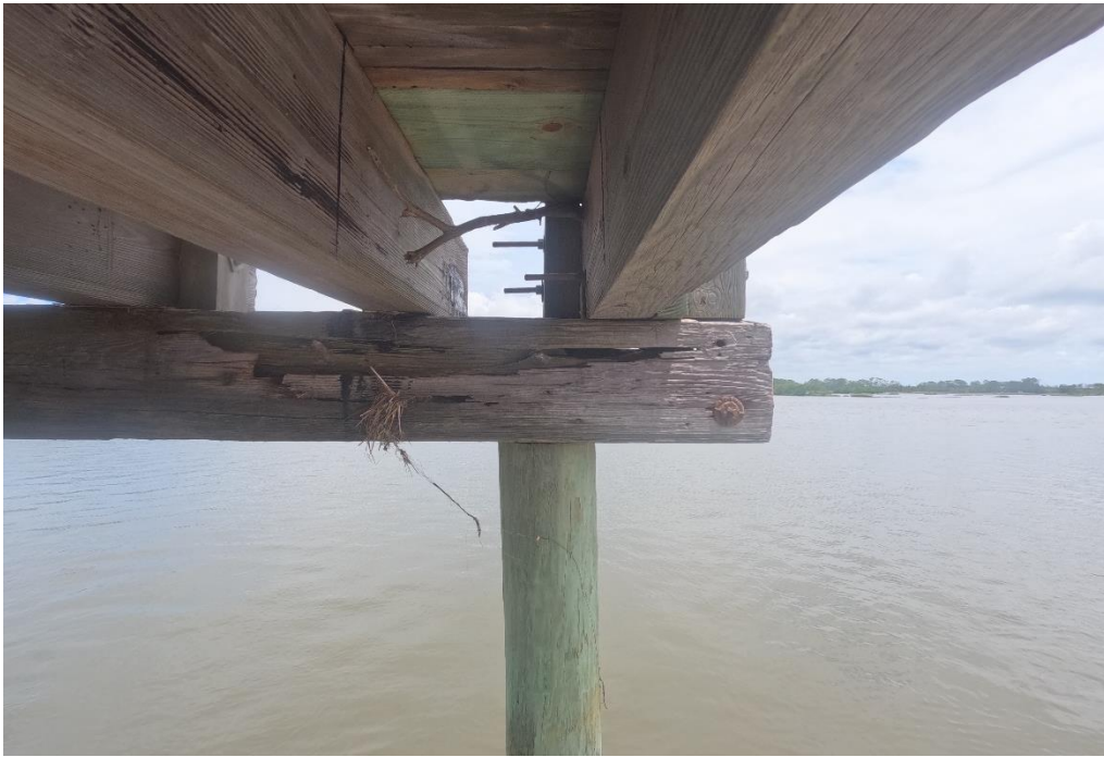
Photo 20: Bent 15. Internal voids within pile cap resulting from fungal decay.
