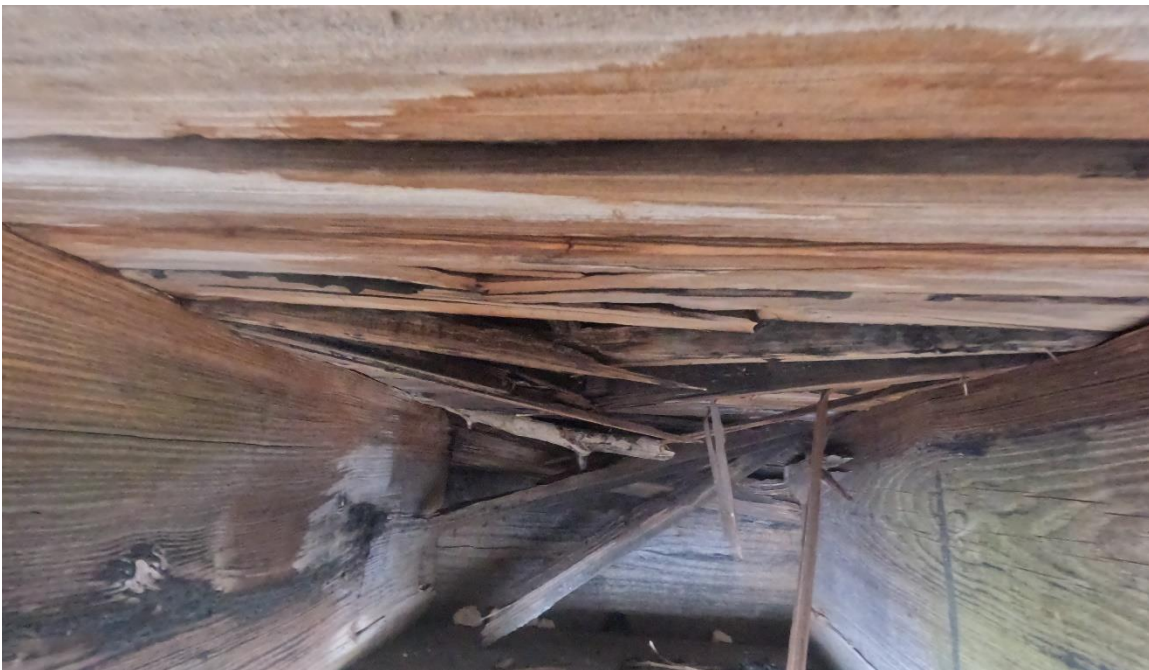
Photo 19: Timber decking failed due to deterioration.
