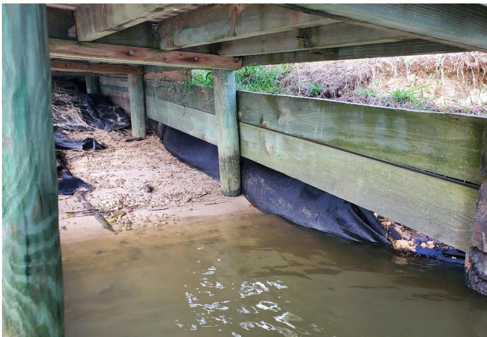
Photo 28: Timber along eastern side of backwall does not extend to mudline resulting in loss of backfill. Note boarding pier piles provide lateral support to backwall timber.
