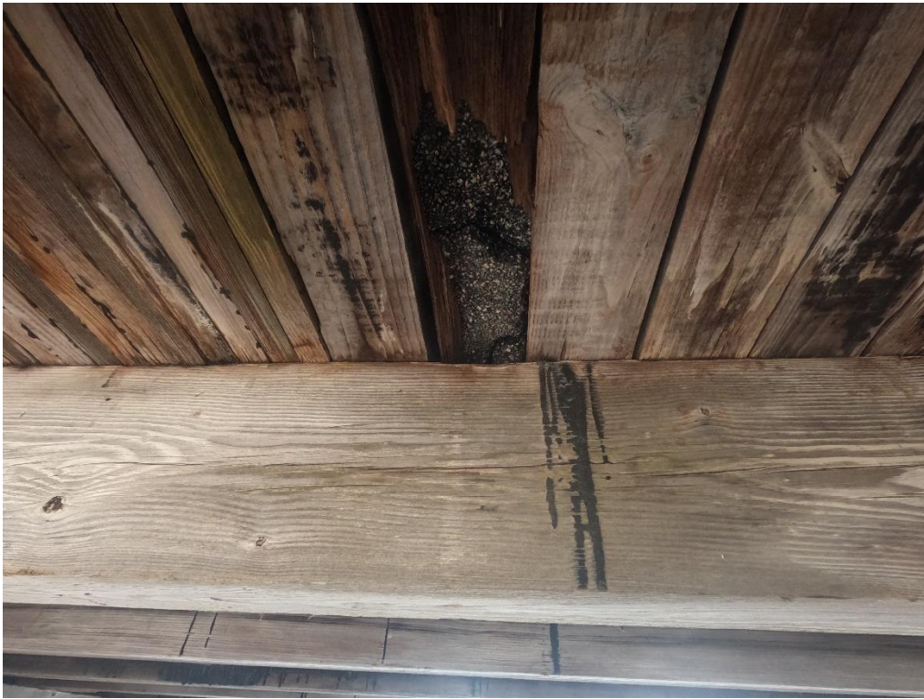
Photo 18: Timber decking deteriorated exposing asphalt overlay.
