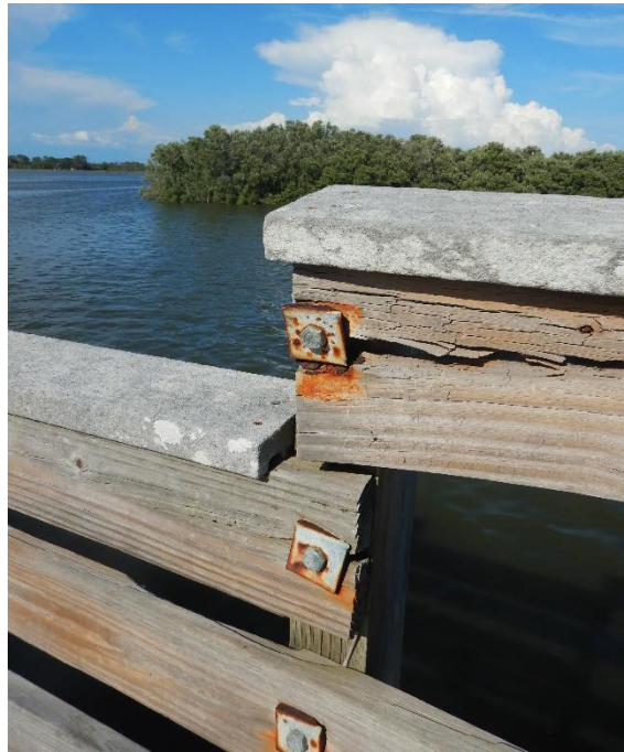
Photo 7: Typical conditions of railing timber and fasteners. Note checks and corroding fasteners.
