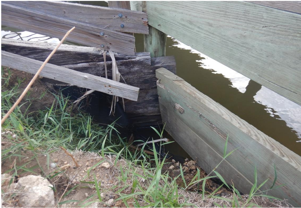
Photo 27: Timber along eastern side of backwall does not extend to mudline resulting in loss of backfill.
