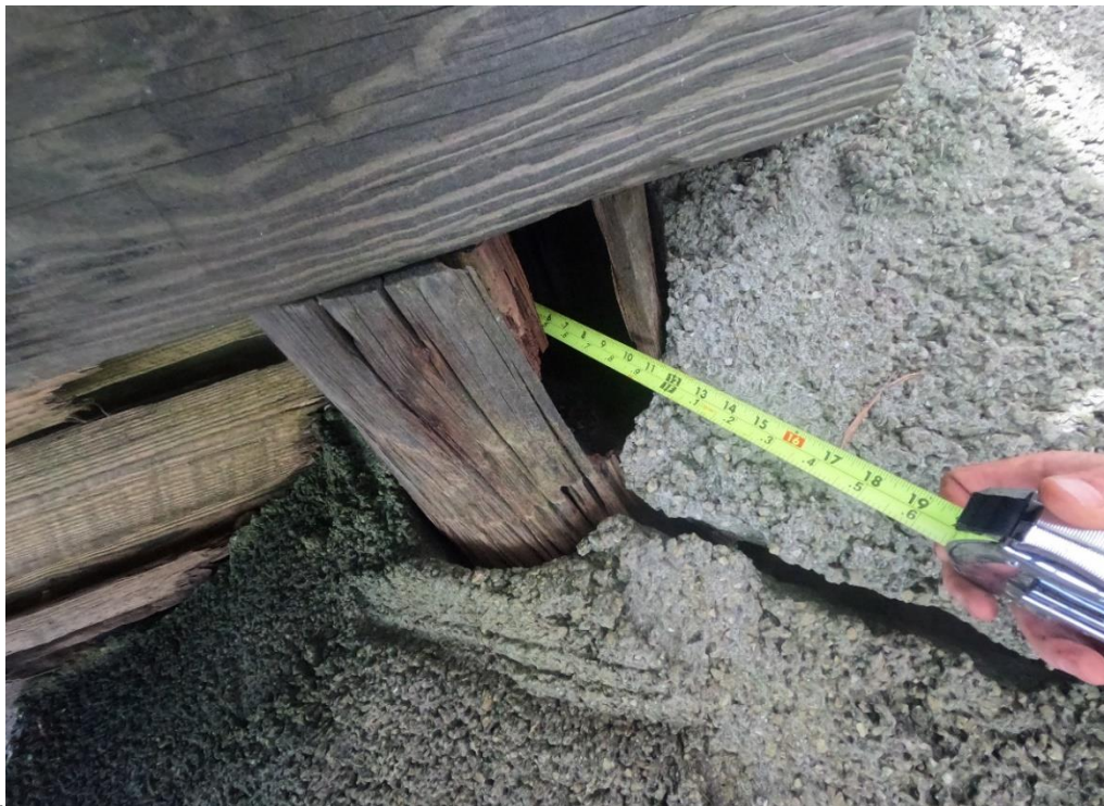
Photo 23 (L) and 24 (R): Pile 1A exhibiting significant loss of section. Inside of pile is completely deteriorated resulting in a 10-inch diameter void. Pile is original.
