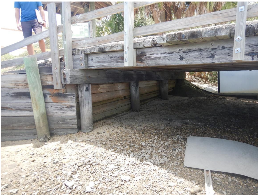
Photo 26: View looking west at backwall. Note multiple layers of timber and the outboard timber exhibiting loss of section caused by marine borer attack.
