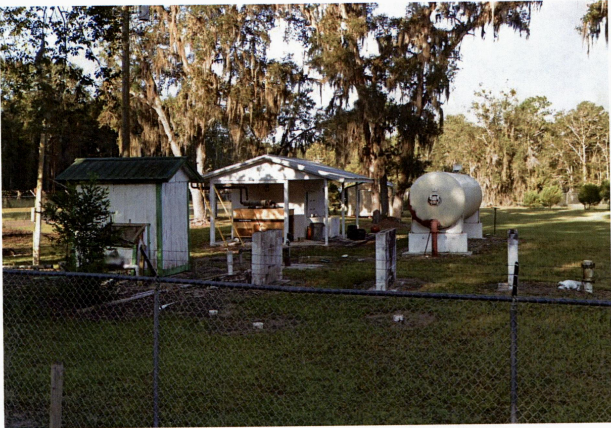
Figure 7: University Oaks WTP looking to the West
