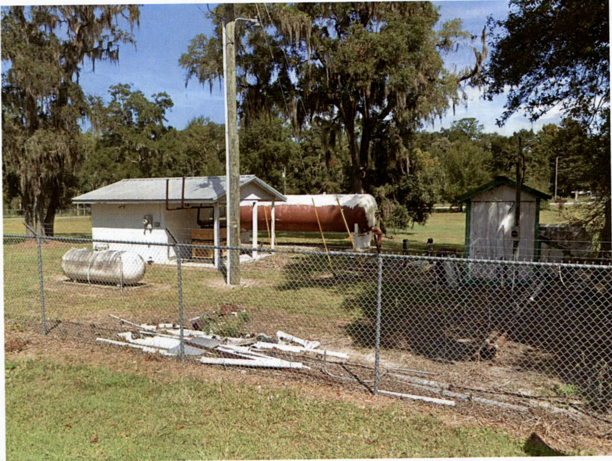
Figure 6: University Oaks WTP looking to the North
