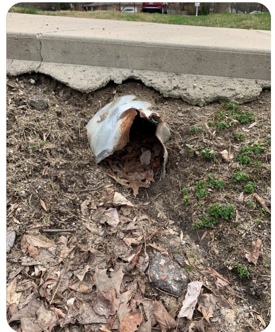
Damaged storm sewer culvert (Giffels Webster)
