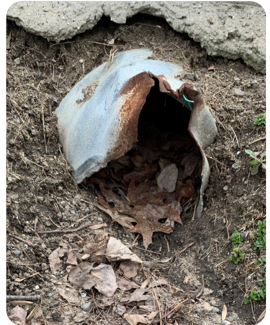
Damaged storm sewer culvert (Giffels Webster)
