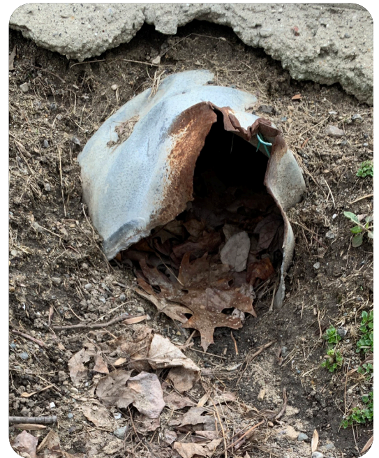
Damaged storm sewer culvert (Giffels Webster)
